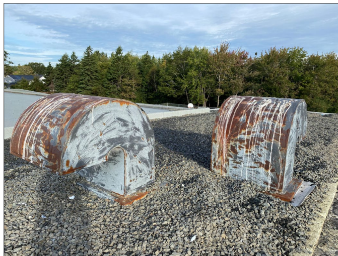
Photo 4 - Two exhaust ducts with asbestos-containing black mastic
