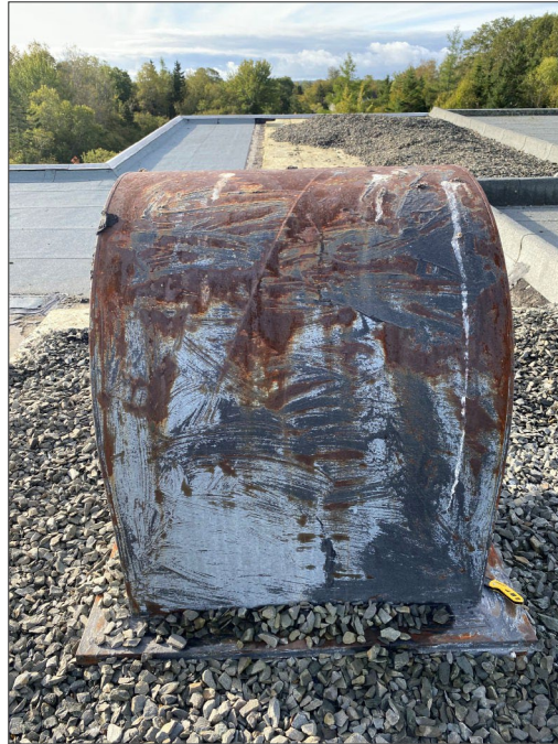
Photo 3 - S0002A-C, Confirmed Asbestos, Black duct mastic
