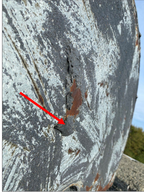
Photo 5 - S0002A-C, Confirmed asbestos, Black mastic
