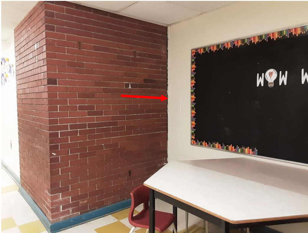
S0028C (Confirmed Asbestos), Black, Wall, Caulking, Hallway (Location #: 40)
