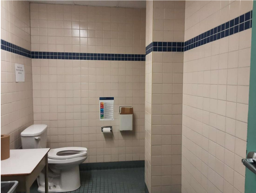
V9500 (Presumed Asbestos), Wall, All, Mortar, Ceramic tile thinset Staff Washroom (Location #: 37)
