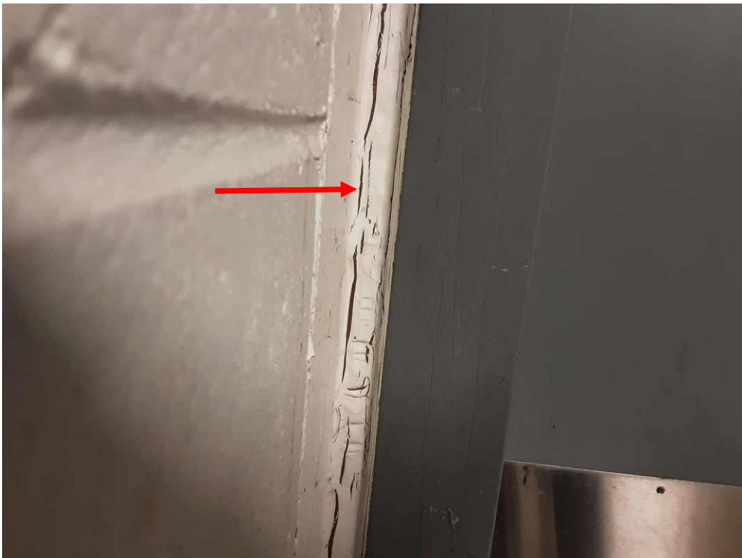
S0007A (Confirmed Asbestos), Brown, Other, Door, Caulking, Basement Entryway (Location #: 4) Painted white
