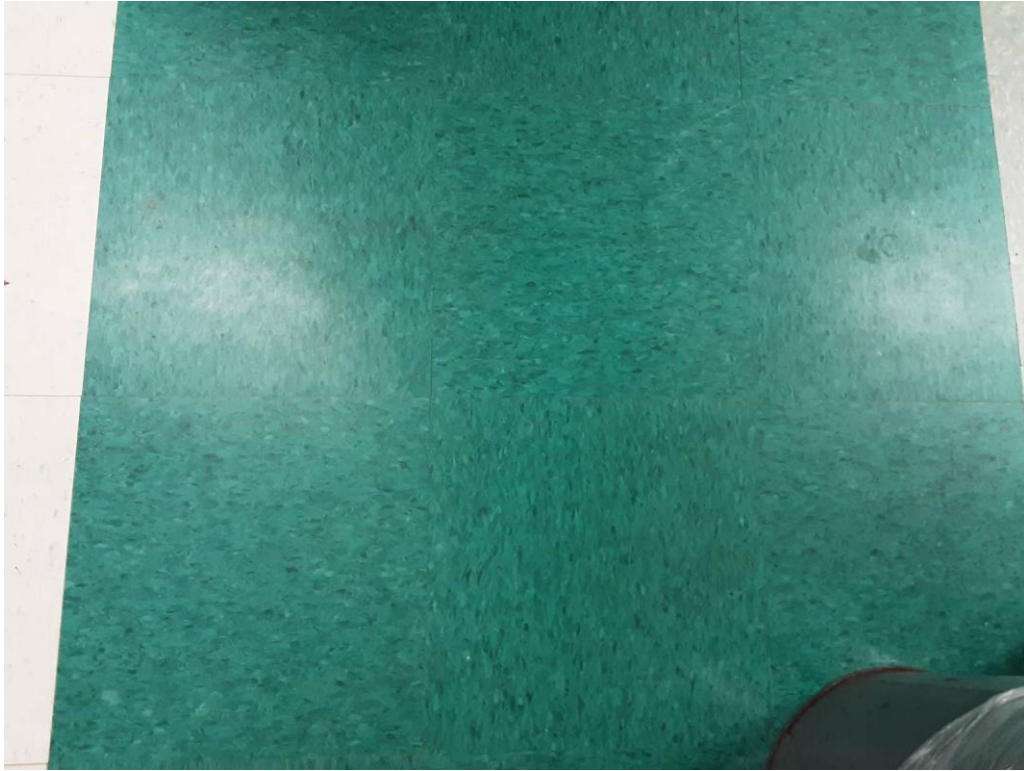
S0013A (Confirmed Asbestos), 12" dark green with flecks, Floor, All, Vinyl Floor Tile and Mastic, Classroom (Location #: 13)
