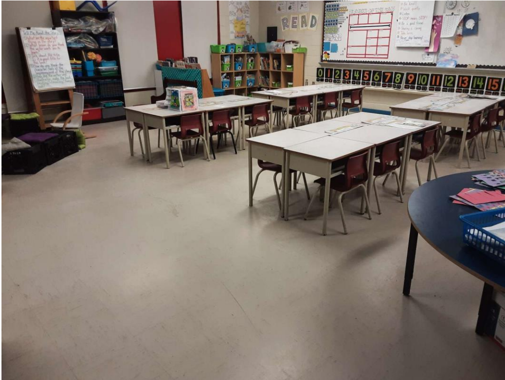
S0015A (Confirmed Asbestos), 12" beige with brown streaks, Floor, All, Vinyl Floor Tile and Mastic, Classroom (Location #: 15)
