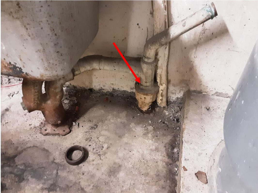
Lead Products, V9000(Yes), BELL AND SPIGOT FITTINGS, Boiler Room (Location #: 1)
