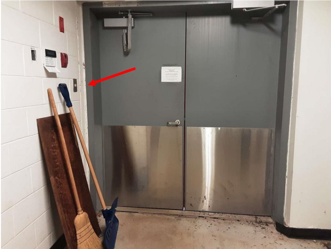
S0007A (Confirmed Asbestos), Brown, Other, Door, Caulking, Basement Entryway (Location #: 4) Painted white
