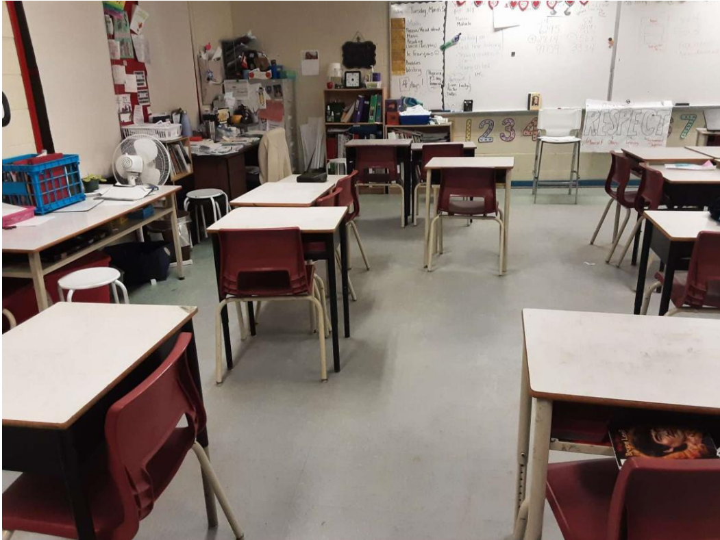
V9000 (Confirmed Asbestos), 12" grey with grey and white flecks, Floor, All, Vinyl Floor Tile and Mastic, Classroom (Location #: 33) Homogenous installation with other flooring present. No discreet area to sample
