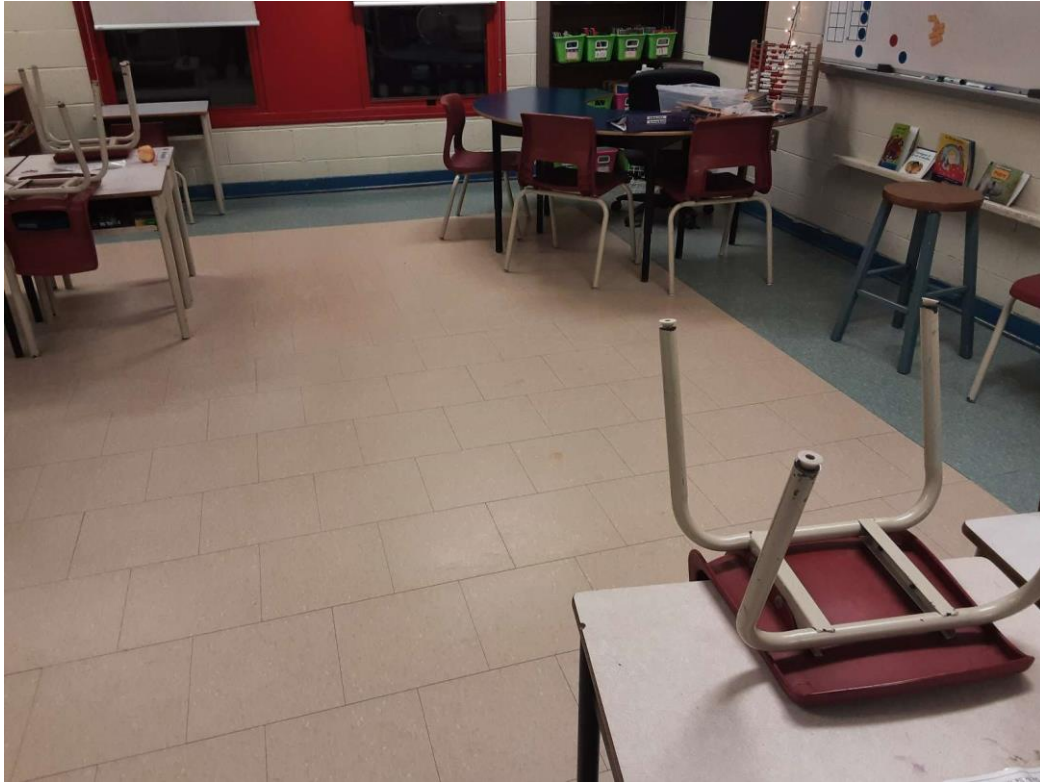
S0017A (Confirmed Asbestos), 12" tan with beige flecks, Floor, All, Vinyl Floor Tile and Mastic, Classroom (Location #: 16)
