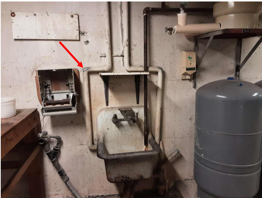
S0002C (Confirmed Asbestos), Piping, Domestic Water (Hot and Cold), Parging Cement, Boiler Room (Location #: 1)
