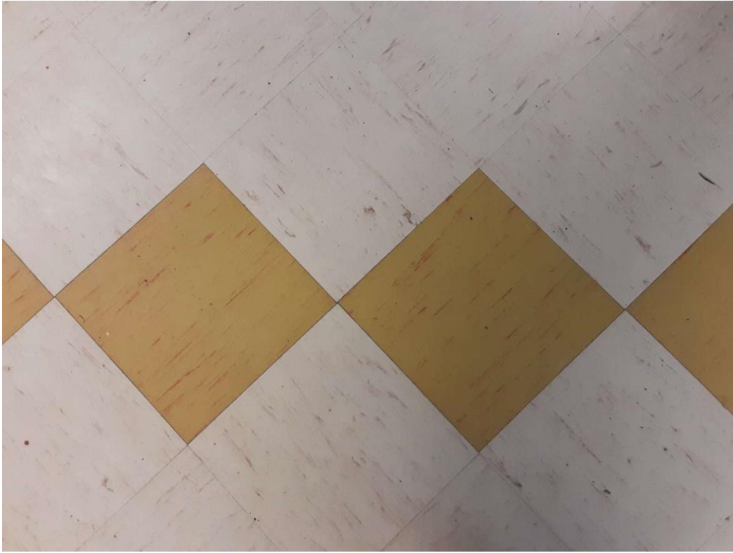
S0027A (Confirmed Asbestos), 12" yellow with red streaks, Floor, All, Vinyl Floor Tile and Mastic, Hallway (Location #: 40)
