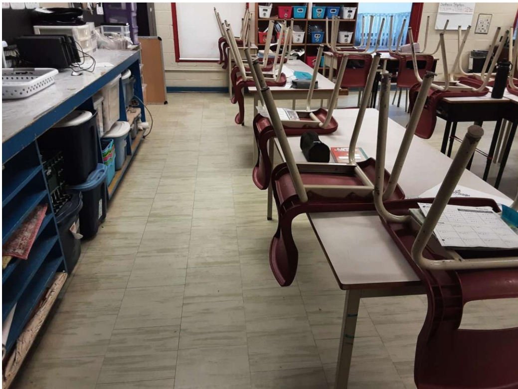
S0029C (Confirmed Asbestos), 12" pale green with light green streaks, Floor, All, Vinyl Floor Tile and Mastic, Classroom (Location #: 46)
