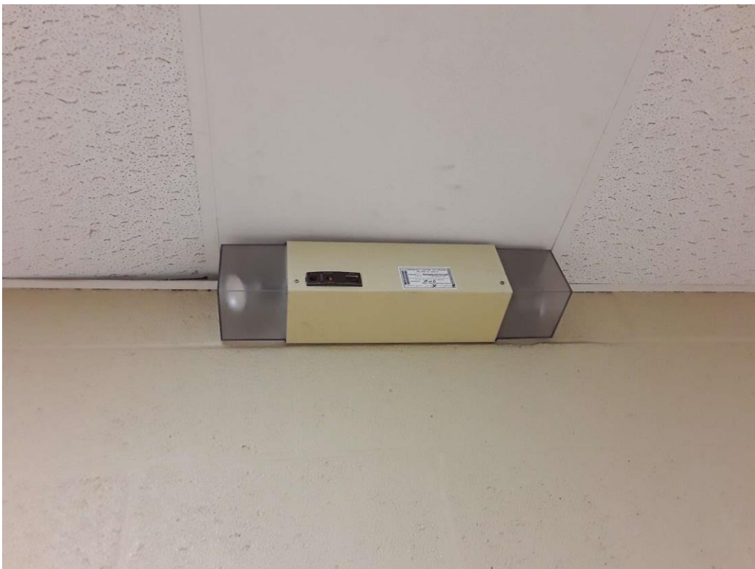
Lead Products, V9500(Presumed), BATTERIES IN EMER. LIGHTS, Hallway (Location #: 47)
