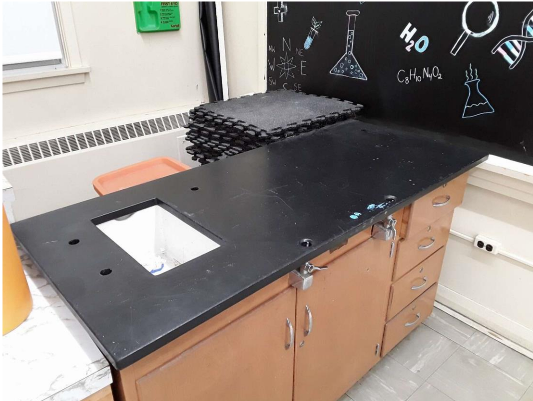
V9500 (Presumed Asbestos), Other, Countertop, Bakelite, Science Lab (Location #: 48)
