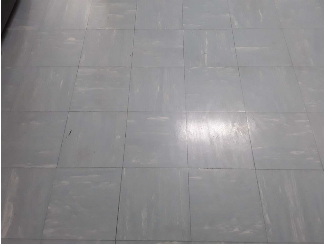
S0010A (Confirmed Asbestos), 12" light blue with white streaks, Floor, Vinyl Floor Tile and Mastic, Office (Location #: 6)
