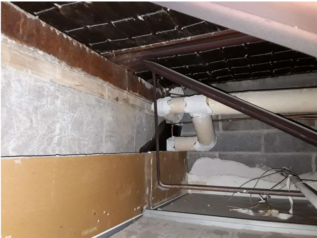
V0003 (Confirmed Asbestos), Piping, Hot Water Heating, Parging Cement, Classroom (Location #: 5)
