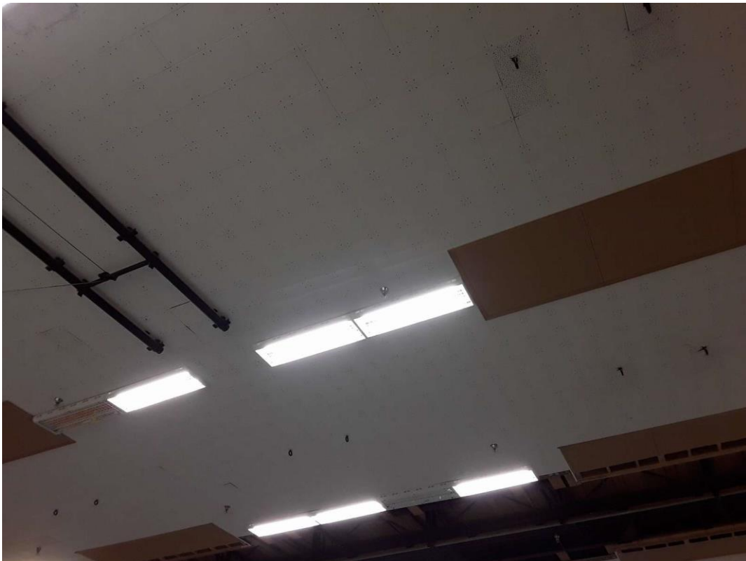
V9500 (Presumed Asbestos), Ceiling, Ceiling tiles (glue-on), Gymnasium (Location #: 26)
