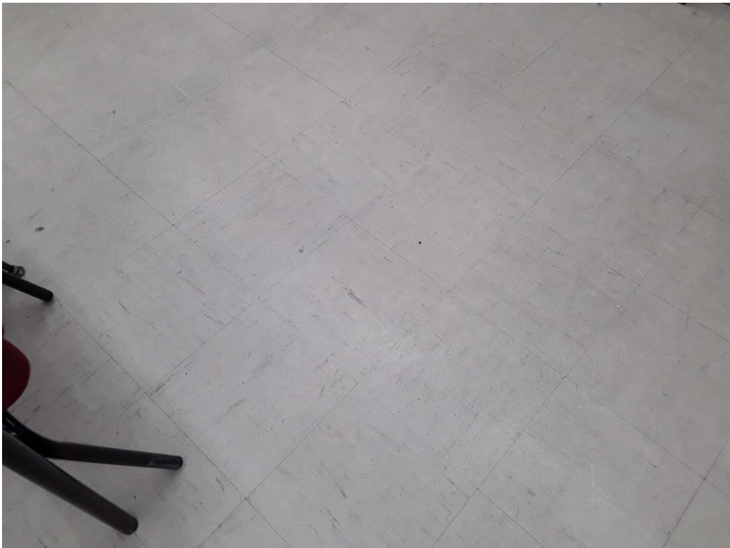
S0017A (Confirmed Asbestos), 12" cream with brown streaks, Floor, Vinyl Floor Tile and Mastic, Classroom (Location #: 25)
