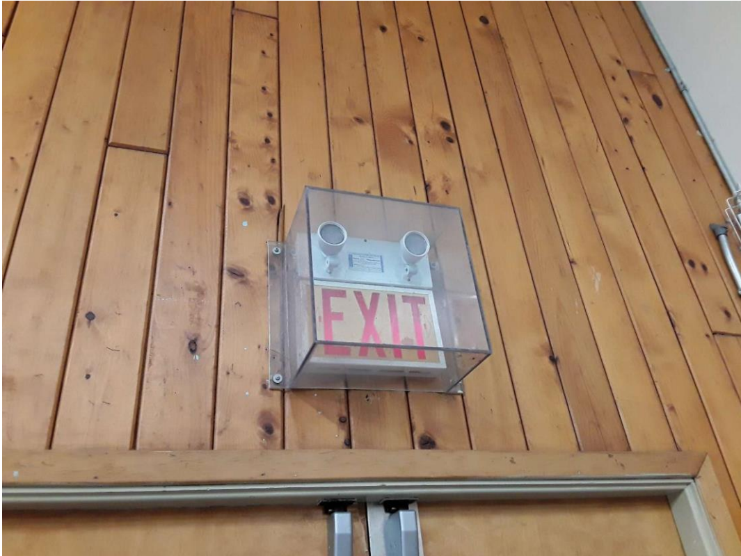
Lead Products, V9500(Presumed), BATTERIES IN EMER. LIGHTS, Gymnasium (Location #: 26)
