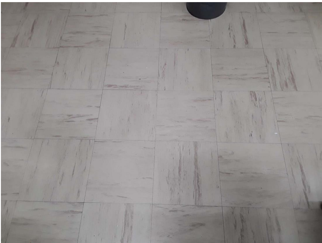
S0030A (Confirmed Asbestos), 12" beige with dark brown streaks, Floor, Vinyl Floor Tile and Mastic, Classroom (Location #: 70)
