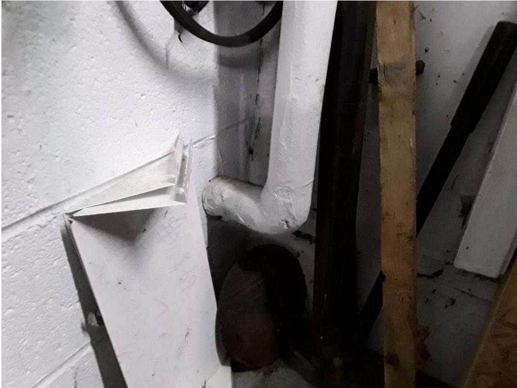
S0003A (Confirmed Asbestos), Piping, Hot Water Heating, Parging Cement, Boiler Room (Location #: 2) Corner by exterior door
