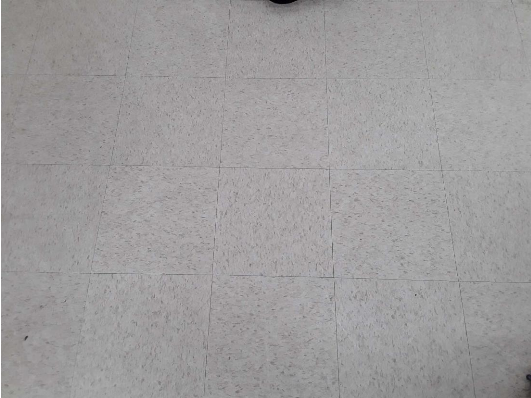
S0006A (Confirmed Asbestos), 12" beige with light brown flecks, Floor, Vinyl Floor Tile and Mastic, Music Room (Location #: 3)
