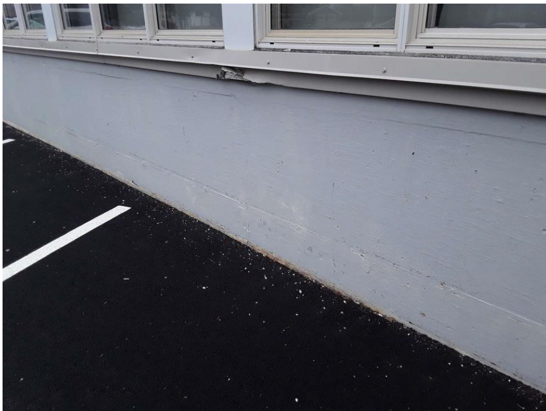
L0001 (Lead, Low), Grey, Structure, Exterior (Location #: 1)
