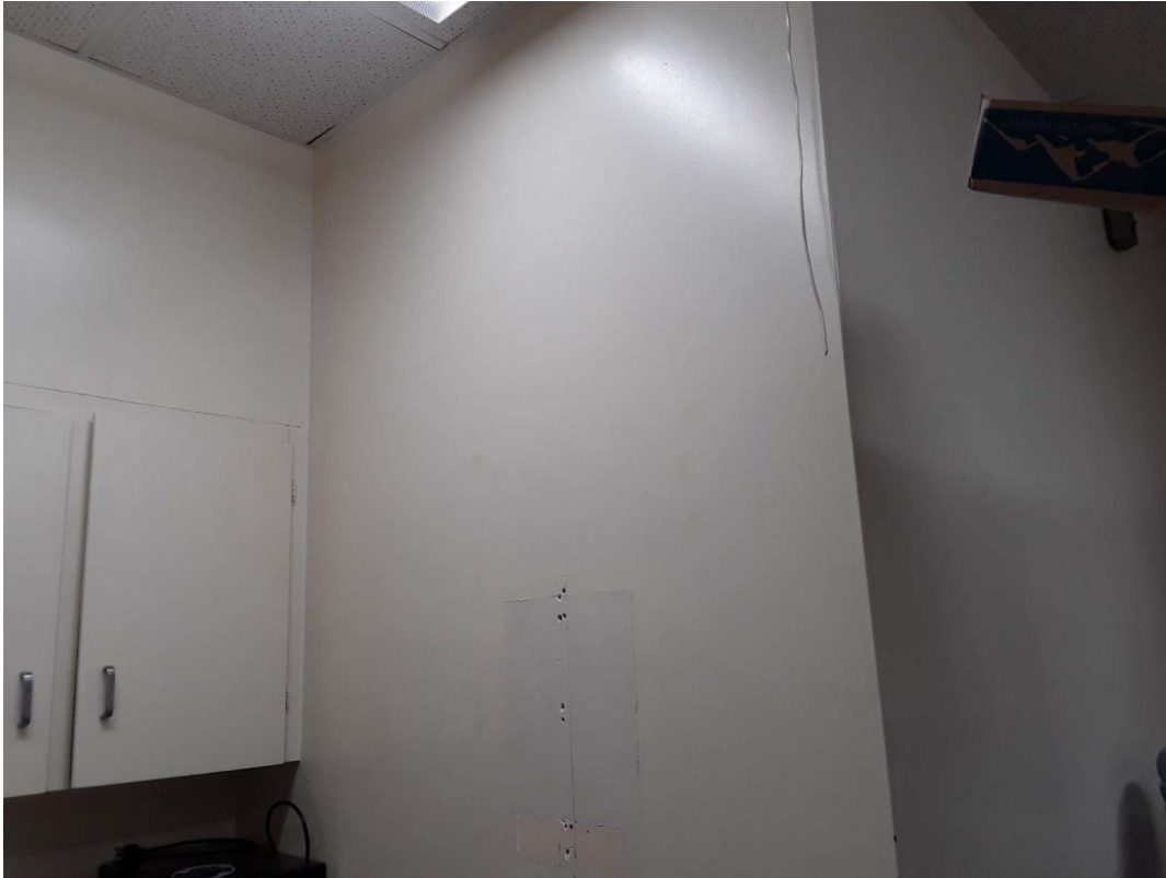
L0006 (Lead, Low), Pale yellow, Wall, Kitchen (Location #: 10)
