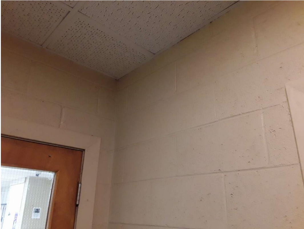
L0009 (Lead, Low), Tan, Wall, Wood Shop Entry (Location #: 37)
