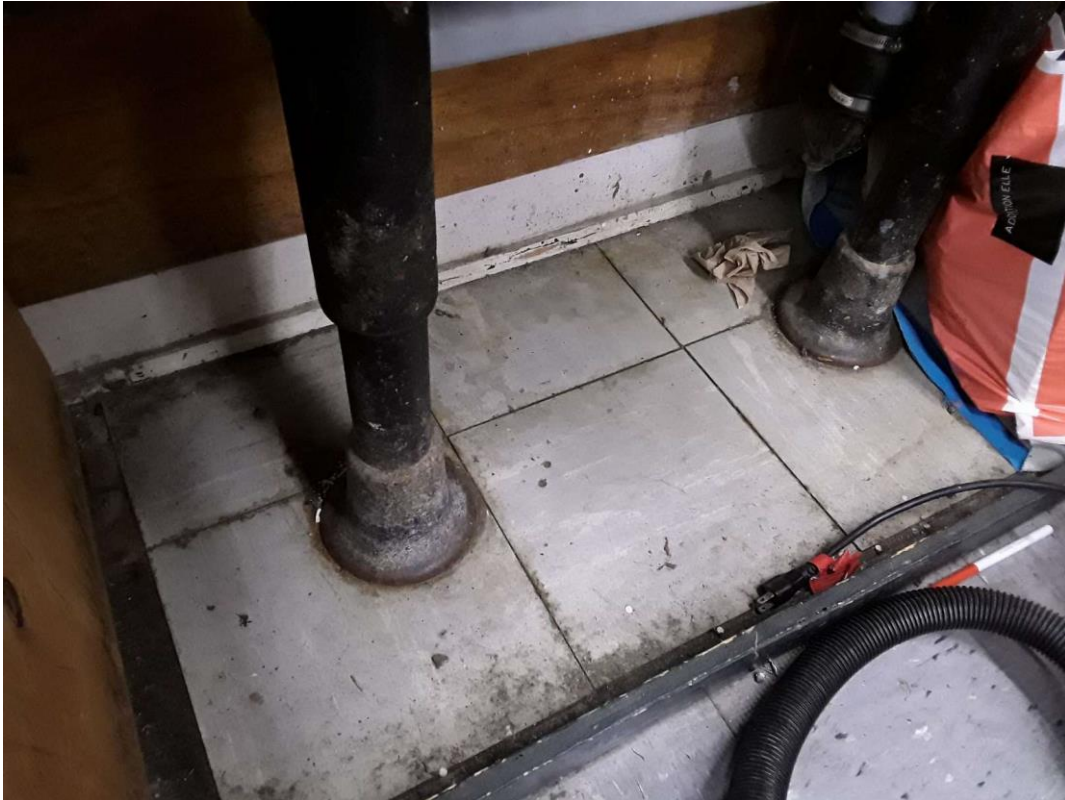
S0021A (Confirmed Asbestos), 12" light grey with white streaks, Floor, Vinyl Floor Tile and Mastic, Band Room (Location #: 39) Under sink
