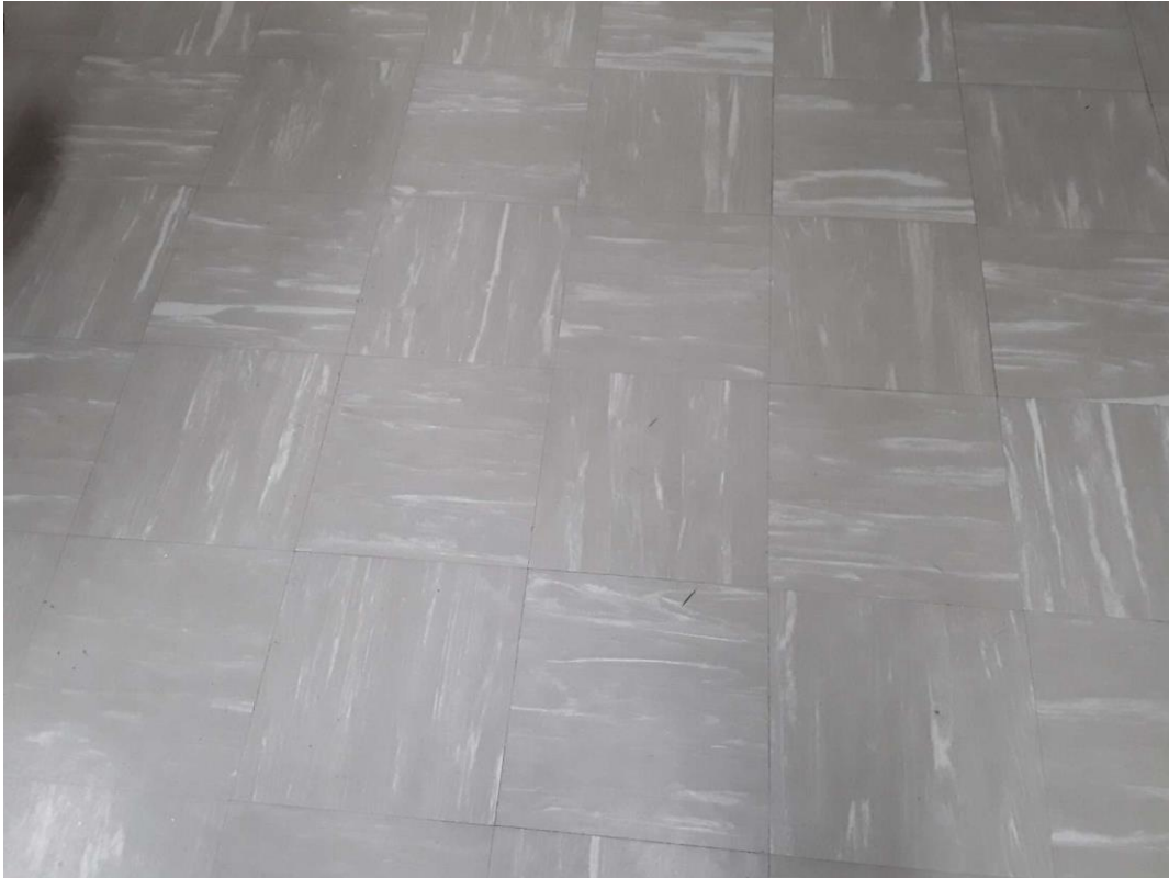
S0016A (Confirmed Asbestos), 12" pale green with light streaks, Floor, Vinyl Floor Tile and Mastic, Library (Location #: 21)
