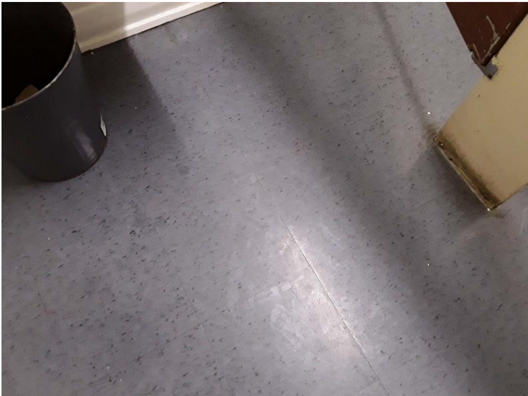
S0015A (Confirmed Asbestos), 12" dark blue with dark flecks, Floor, Vinyl Floor Tile and Mastic, Men's Washroom (Location #: 12)
