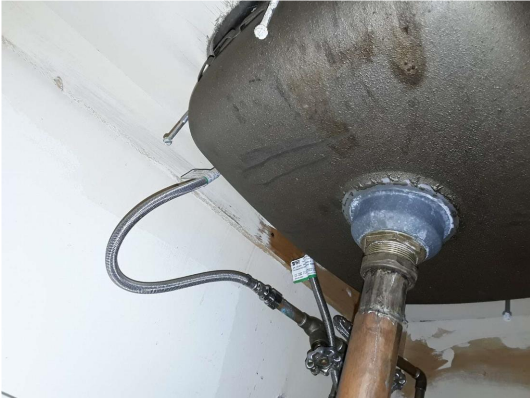
S0014 (Confirmed Asbestos), Other, Sink, Mastic, Gold, Kitchen (Location #: 10)
