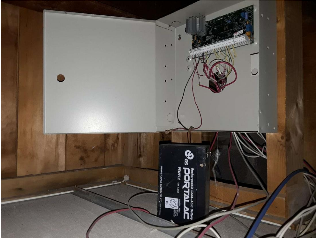
Lead Products, V9000(Yes), BATTERIES (OTHER), Hallway (Location #: 47)
