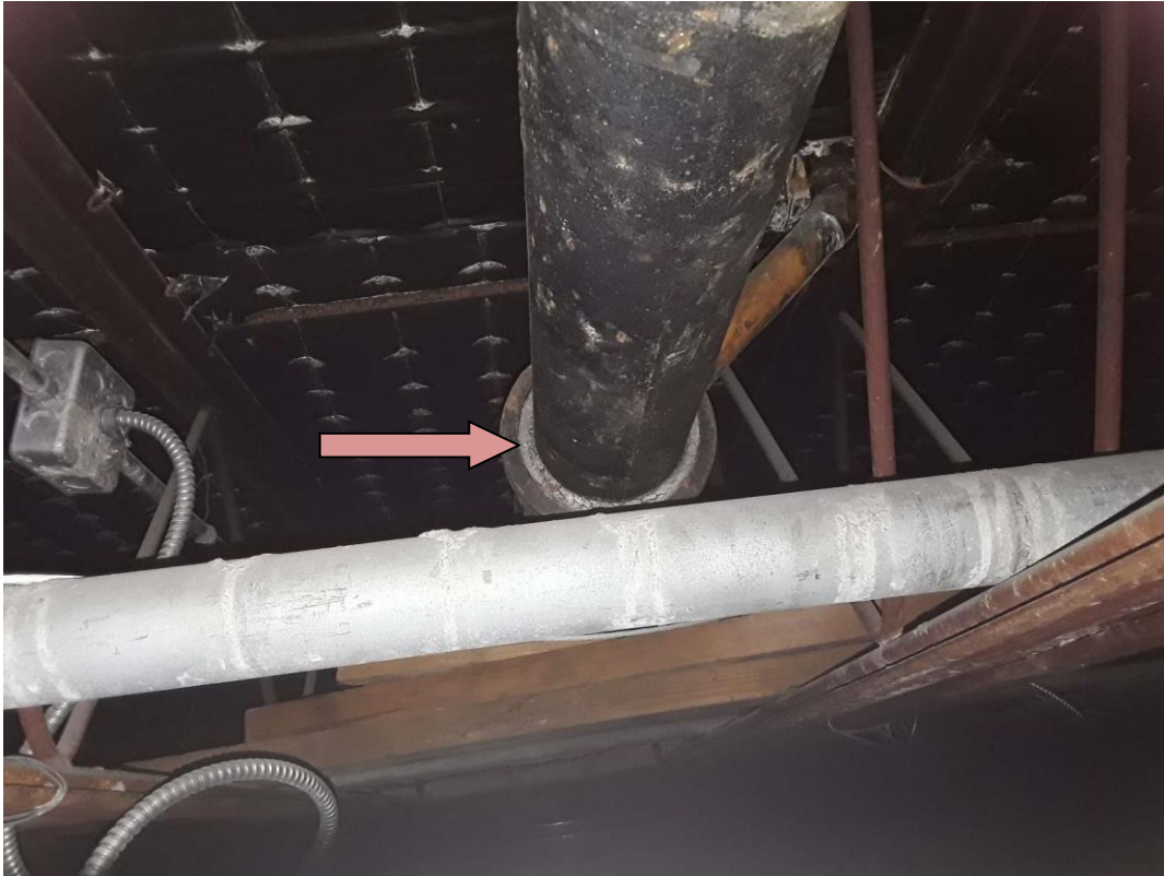
Lead Products, V9000(Yes), BELL AND SPIGOT FITTINGS, Music Room (Location #: 3)
