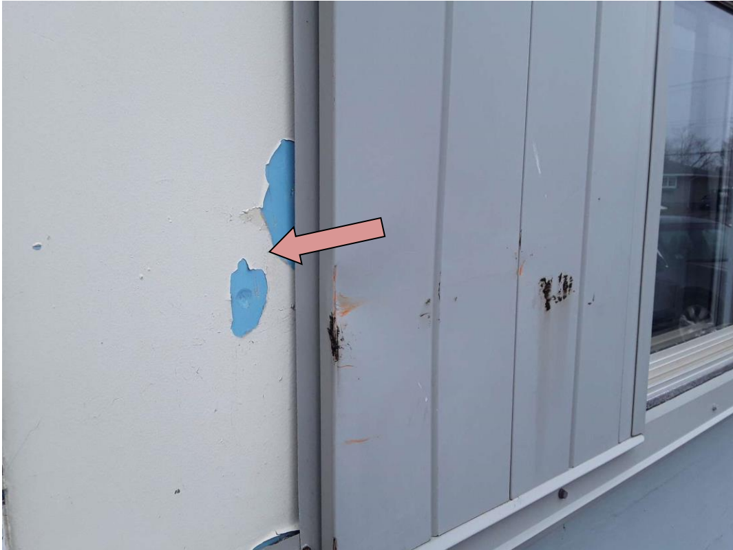
V9500 (Presumed Asbestos), Wall, Cement Product, Exterior (Location #: 1) Visible during the assessment because of a missing panel of metal cladding.
