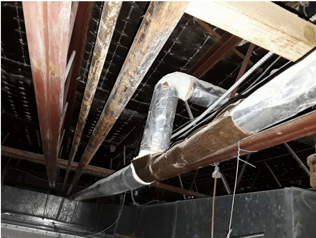
V0011 (Confirmed Asbestos), Piping, Domestic Water (Hot and Cold), Parging Cement, Girls Washroom (Location #: 20)
