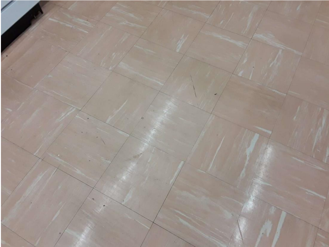
S0027A (Confirmed Asbestos), 12" pink with white streaks, Floor, Vinyl Floor Tile and Mastic, Breakfast Room (Location #: 64)
