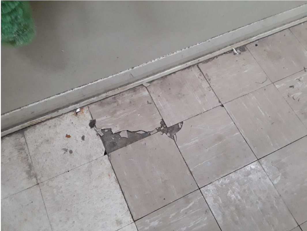
S0012A (Confirmed Asbestos), 12" pale brown with beige streaks, Floor, Vinyl Floor Tile and Mastic, Janitor Room (Location #: 8)
