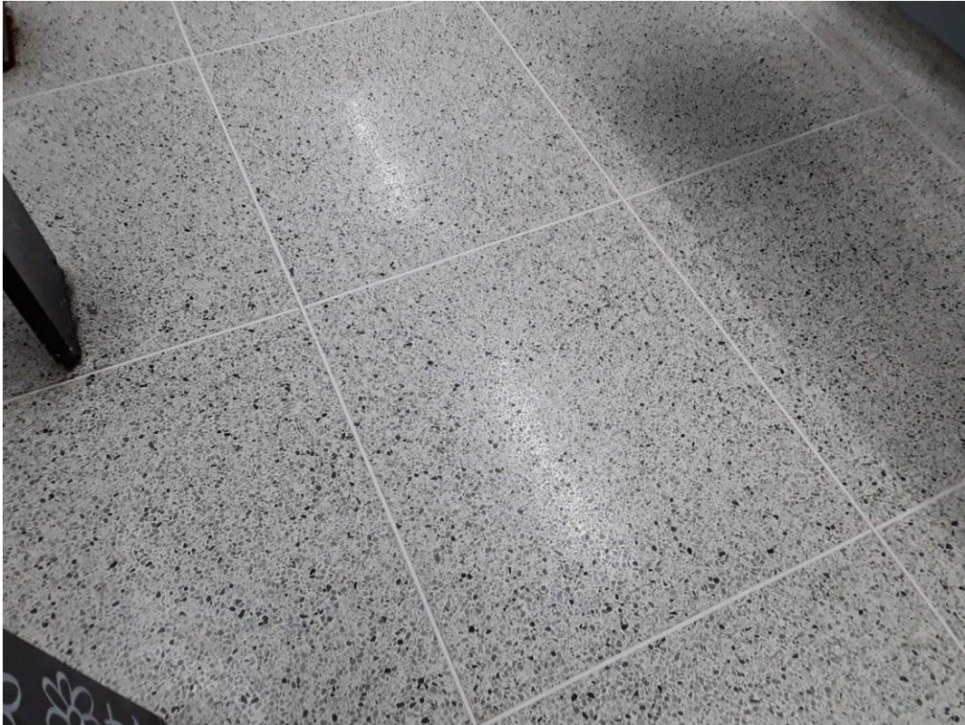
V9500 (Presumed Asbestos), Floor, Terrazzo, Boys Washroom (Location #: 19)
