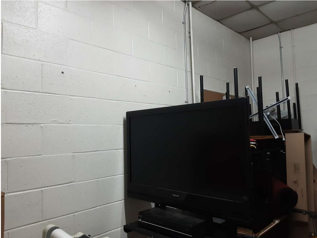
L0003 (Lead, High), White, Wall, Storage Room (Location #: 2)
