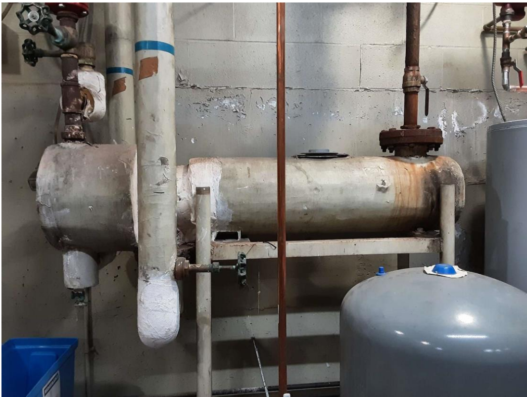
S0003C (Confirmed Asbestos), Mechanical Equipment, Tank, Parging Cement, Boiler Room (Location #: 1)
