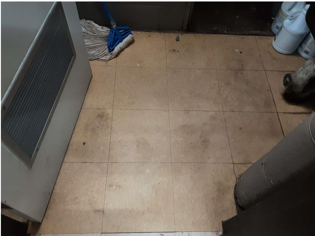
S0018A (Confirmed Asbestos), 12" light brown with flecks, Floor, All, Vinyl Floor Tile and Mastic, Janitor Closet And Pipe Chase (Location #: 26), Asbestos detected in floor mastic
