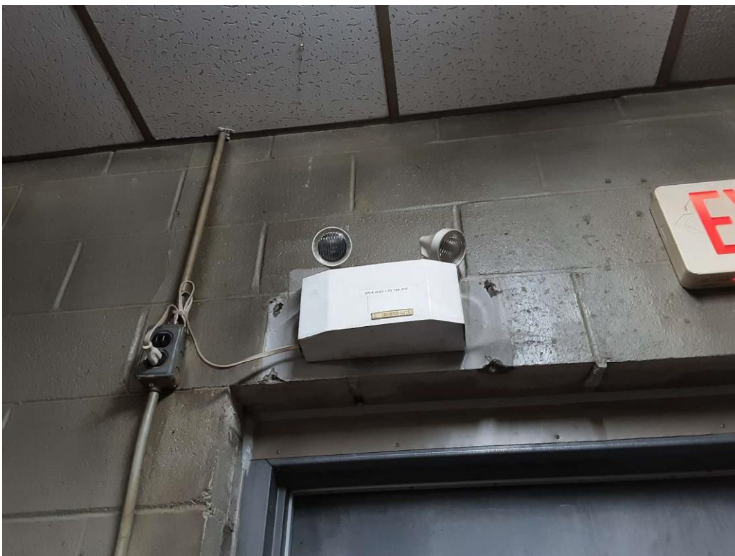
Lead Products, V9500(Presumed), Batteries in Emer. Lights, Boiler Room (Location #: 1)
