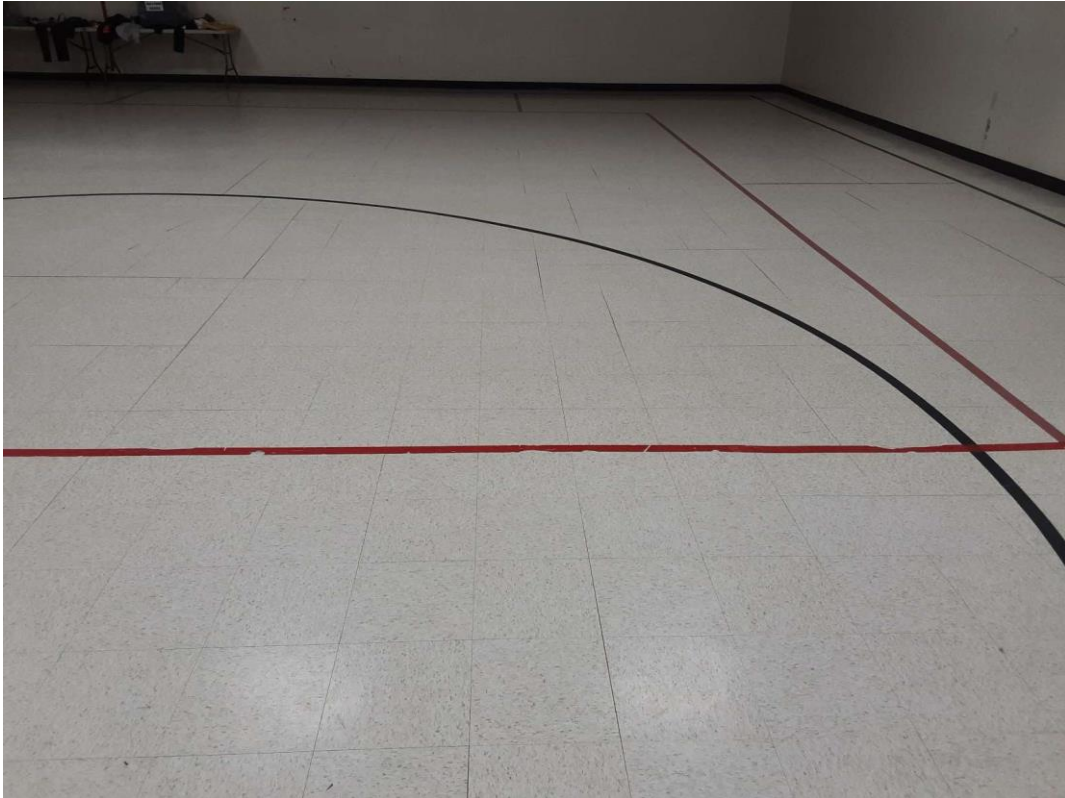
V0007 (Confirmed Asbestos), 12" off-white with beige and cream flecks, Floor, All, Vinyl Floor Tile and Mastic, Gym And Stage (Location #: 52), Asbestos detected in floor mastic
