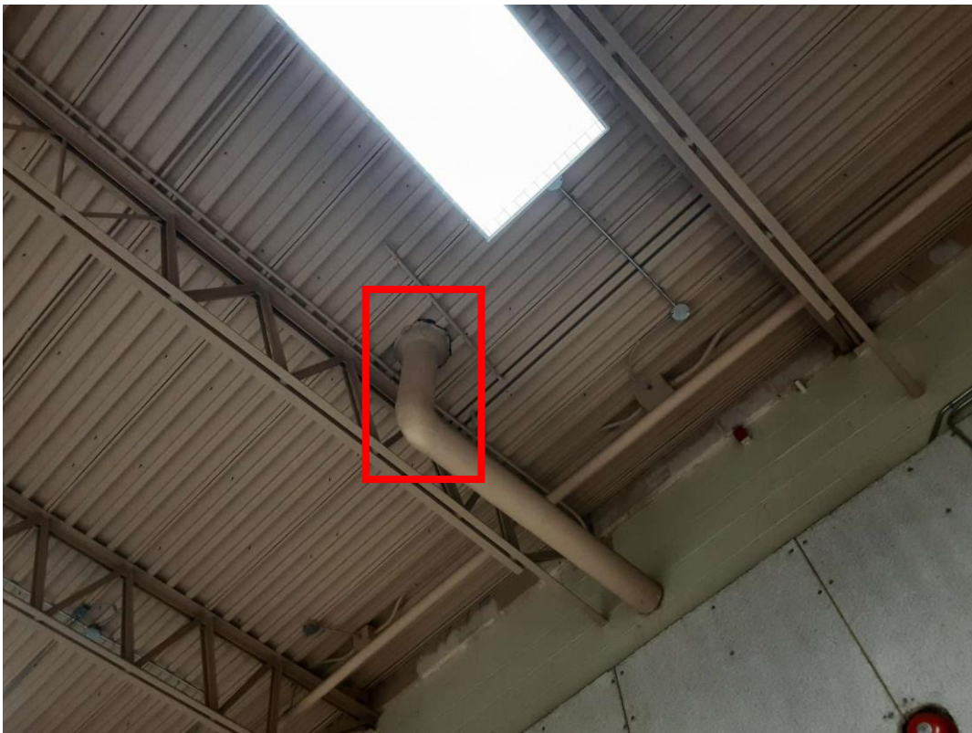
V9500 (Presumed Asbestos), Piping, Roof Hopper (Drain), Parging Cement, Gym And Stage (Location #: 52)
