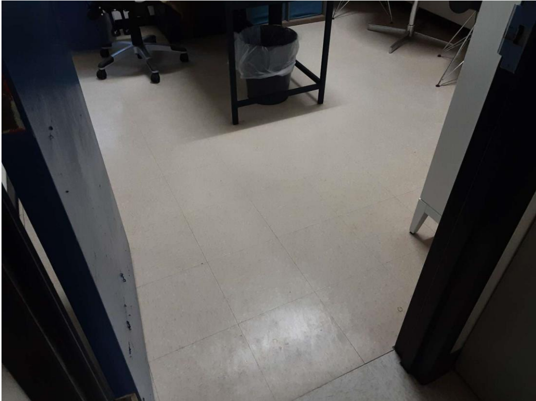
S0004A (Confirmed Asbestos), 12" cream with beige and white flecks, Floor, All, Vinyl Floor Tile and Mastic, Office (Location #: 3), Asbestos detected in floor mastic
