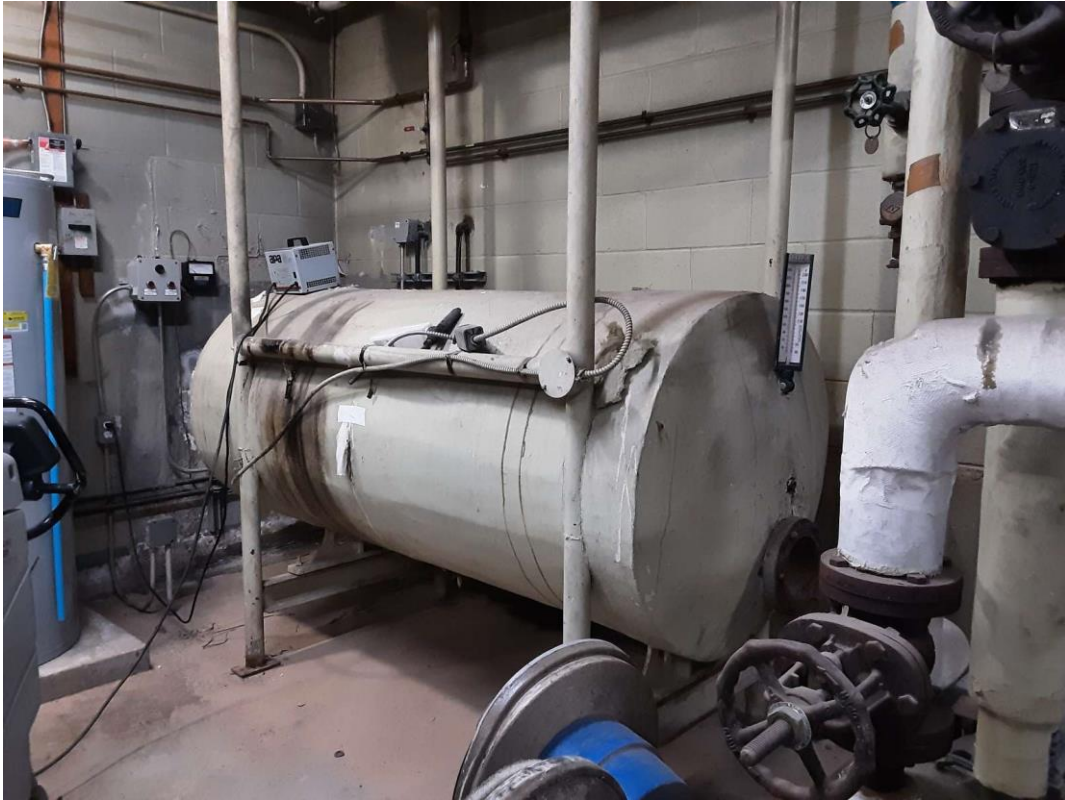
S0002C (Confirmed Asbestos), Mechanical Equipment, Heating Water Tank, Parging cement and Preformed Block, Boiler Room (Location #: 1)
