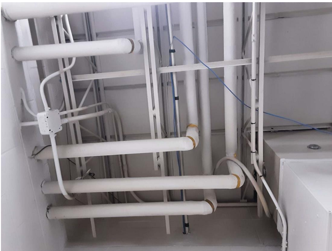
S0009A (Confirmed Asbestos), Piping, Domestic Water (Hot and Cold), Parging Cement, Storage Room (Location #: 9) Good condition
