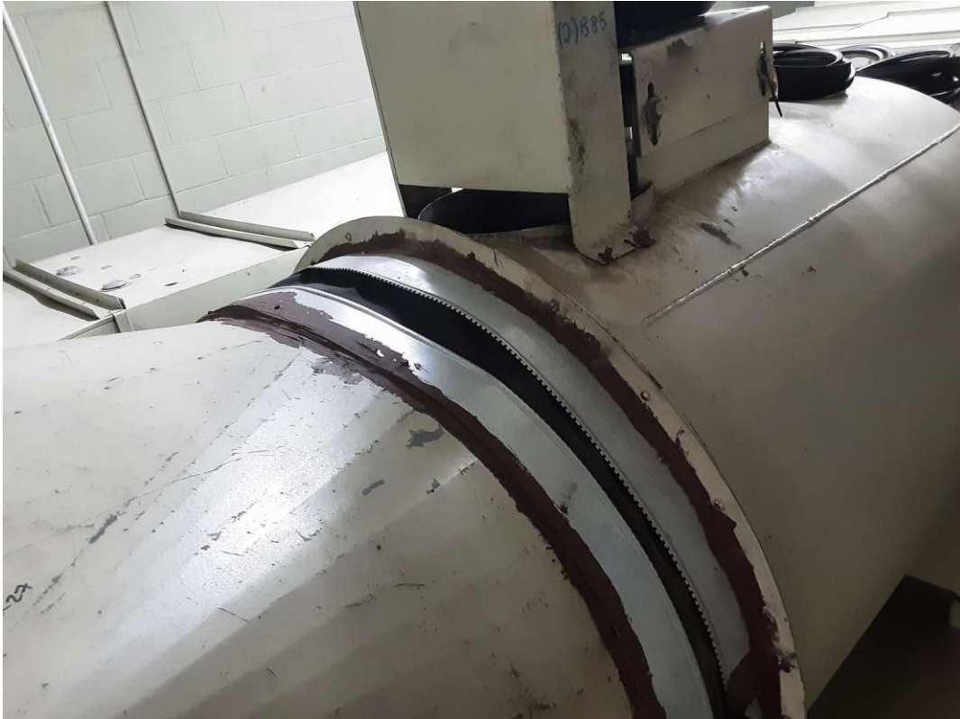
S0017C (None), Duct, Supply Air, Mastic, Red, Mechanical Room (Location #: 23)
