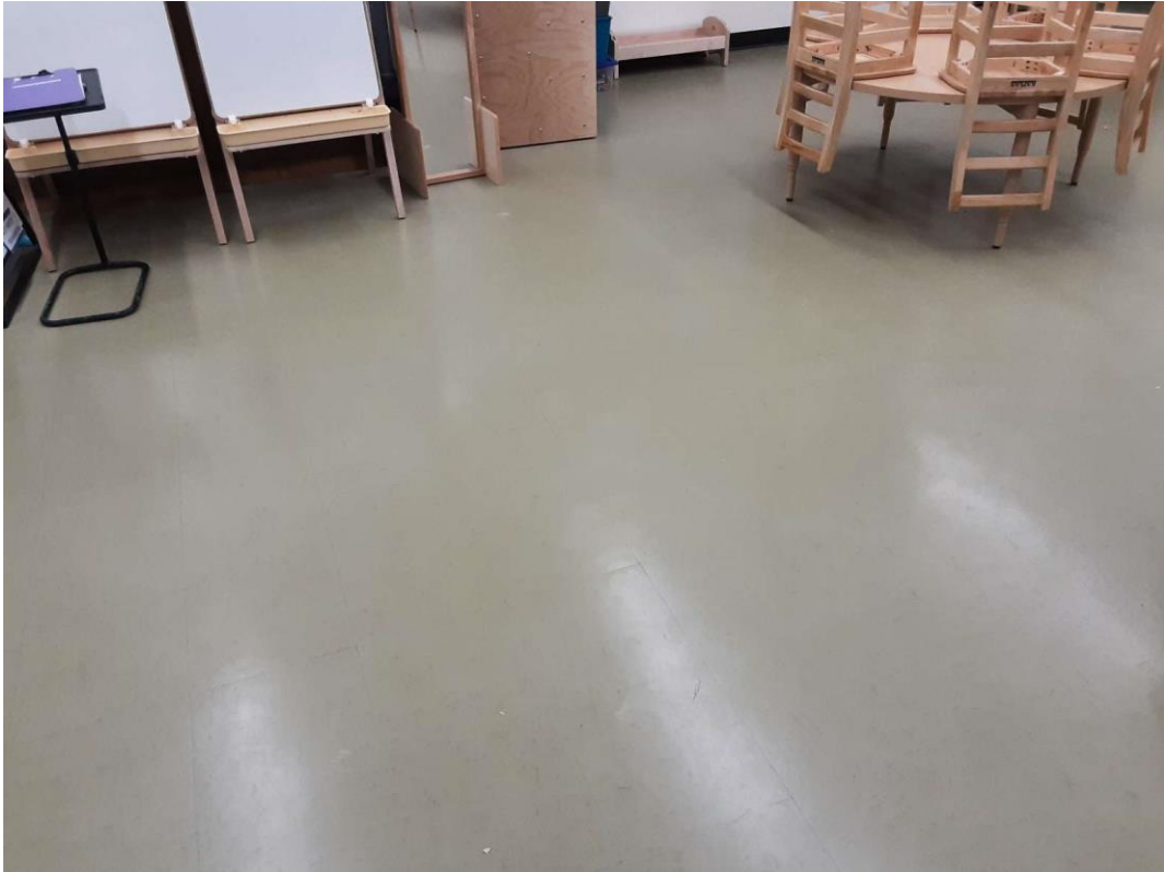
S0013B (Confirmed Asbestos), 12" forest green with faint brown streaks, Floor, All, Vinyl Floor Tile and Mastic, Classroom (Location #: 15), Asbestos detected in vinyl tile and mastic
