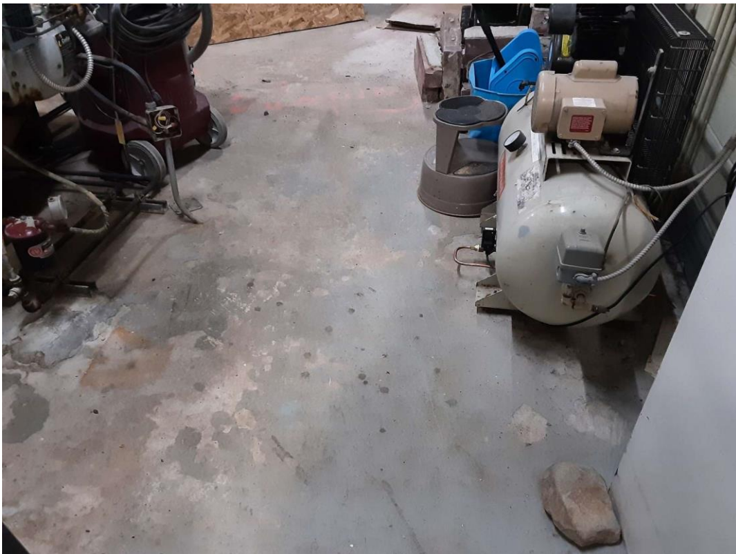
L0002 (Lead, High), Grey, Floor, Boiler Room (Location #: 1)
