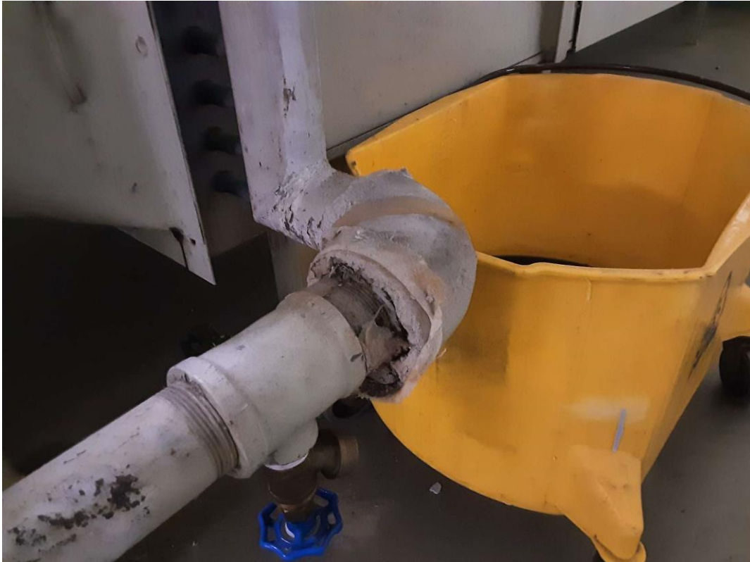
S0009C (Confirmed Asbestos), Piping, Domestic Water (Hot and Cold), Parging Cement, Mechanical Room (Location #: 23)
