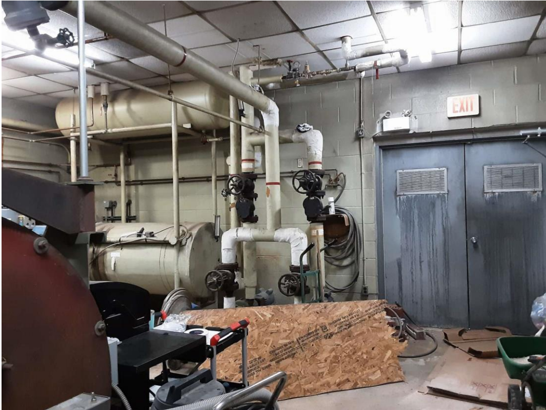
L0001 (Lead, High), Green, Wall, Boiler Room (Location #: 1)
