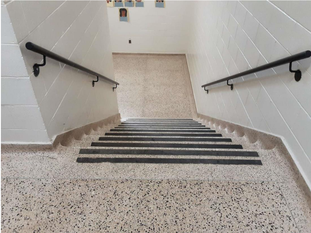
V9500 (Presumed Asbestos), Floor, All, Terrazzo, East Stairwell (Location #: 50)
