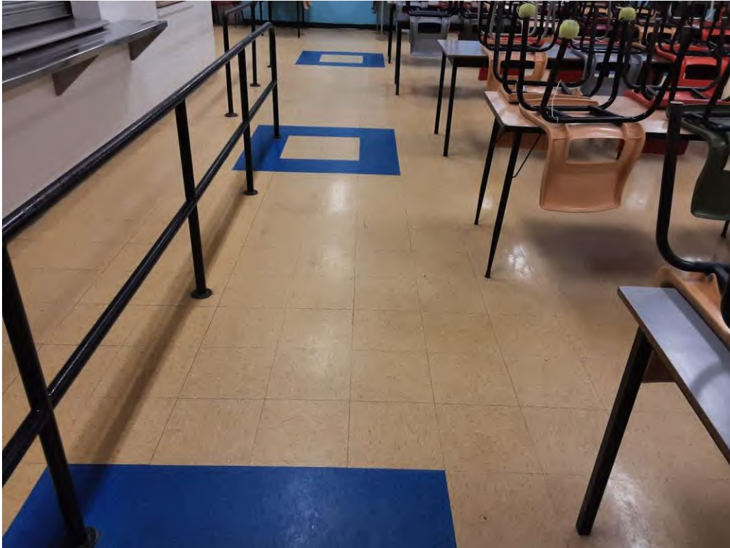
S0023B (Confirmed Asbestos), 12" yellow with flecks, Floor, All, Vinyl Floor Tile and Mastic, Cafeteria (Location #: 41)
