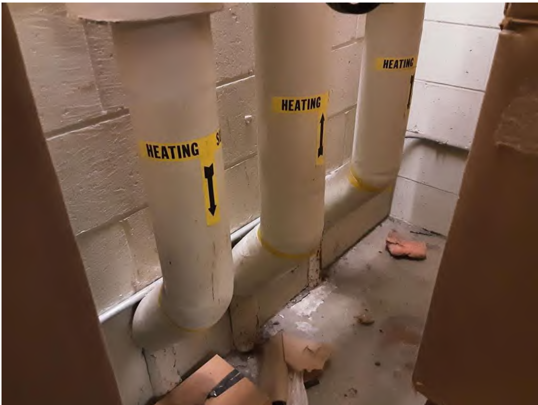
S0001B (Confirmed Asbestos), Piping, Heating Water Supply, Parging Cement, Mechanical Room (Location #: 64)
