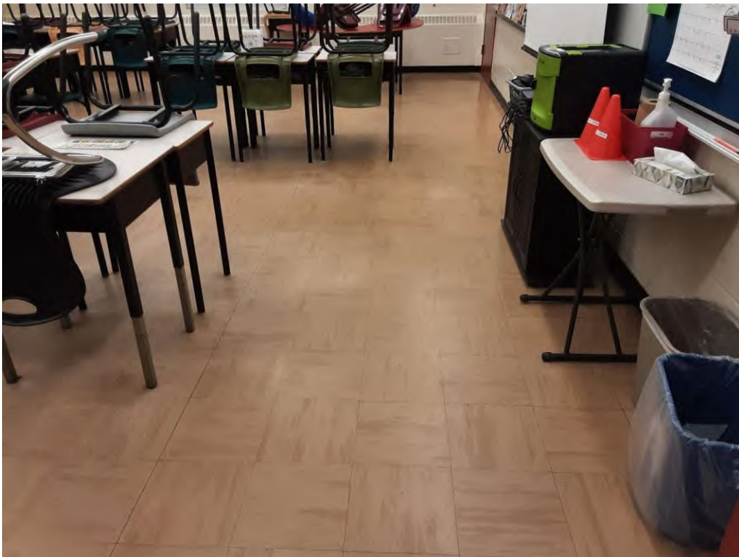
S0024A (Confirmed Asbestos), 12" light brown with brown streaks, Floor, All, Vinyl Floor Tile and Mastic, Classroom (Location #: 51)
