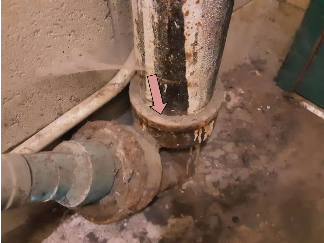
Pb Products, V9000(Yes), BELL AND SPIGOT FITTINGS, Janitor Room (Location #: 19)
