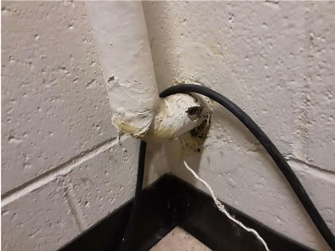
S0002B (Confirmed Asbestos), Piping, Domestic Water (Hot and Cold), Parging Cement, Caretaker Office (Location #: 10)
