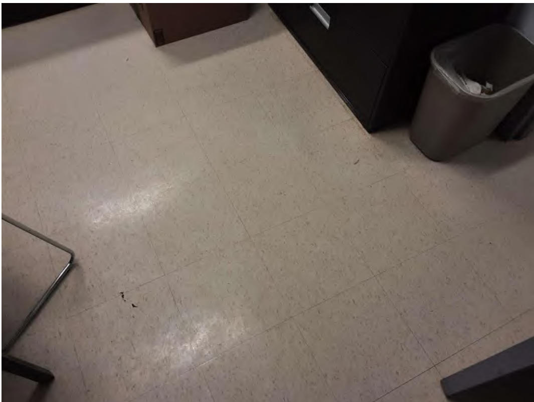
S0009A (Confirmed Asbestos), 12" cream with beige flecks, Floor, All, Vinyl Floor Tile and Mastic, Principal Office (Location #: 4)
