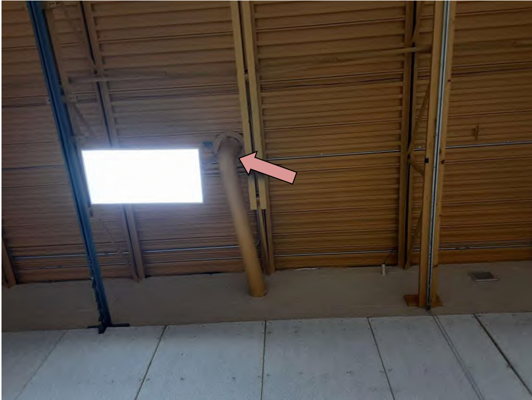
V9500 (Presumed Asbestos), Piping, Drain, Parging Cement, Gym And Stage (Location #: 28)
