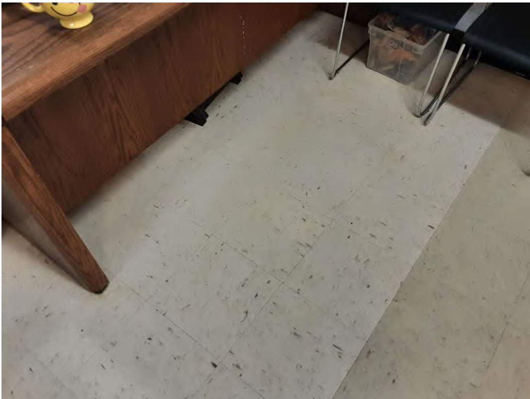
S0012A (Confirmed Asbestos), 12" white with grey flecks, Floor, All, Vinyl Floor Tile and Mastic, Administration Office (Location #: 7)
