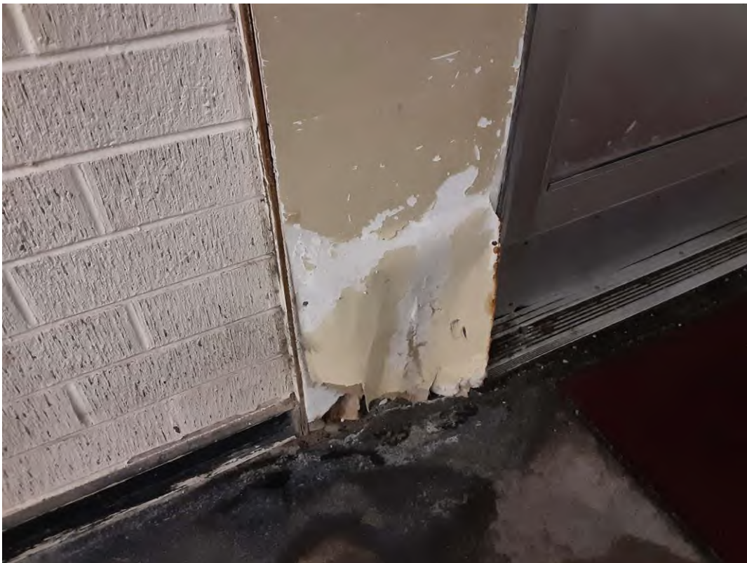
S0007B (Confirmed Asbestos), Wall, Exterior, Drywall and joint compound, Back Vestibule (Location #: 22)
