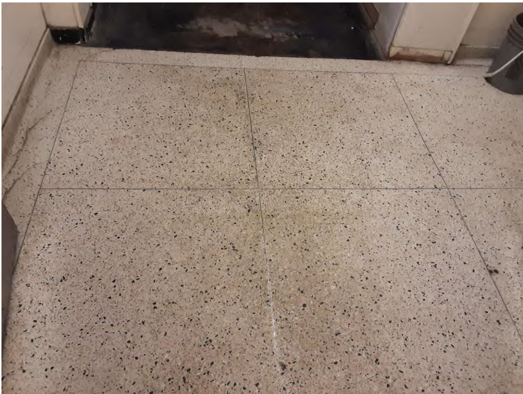
V9500 (Presumed Asbestos), Floor, All, Terrazzo, Back Vestibule (Location #: 22)
