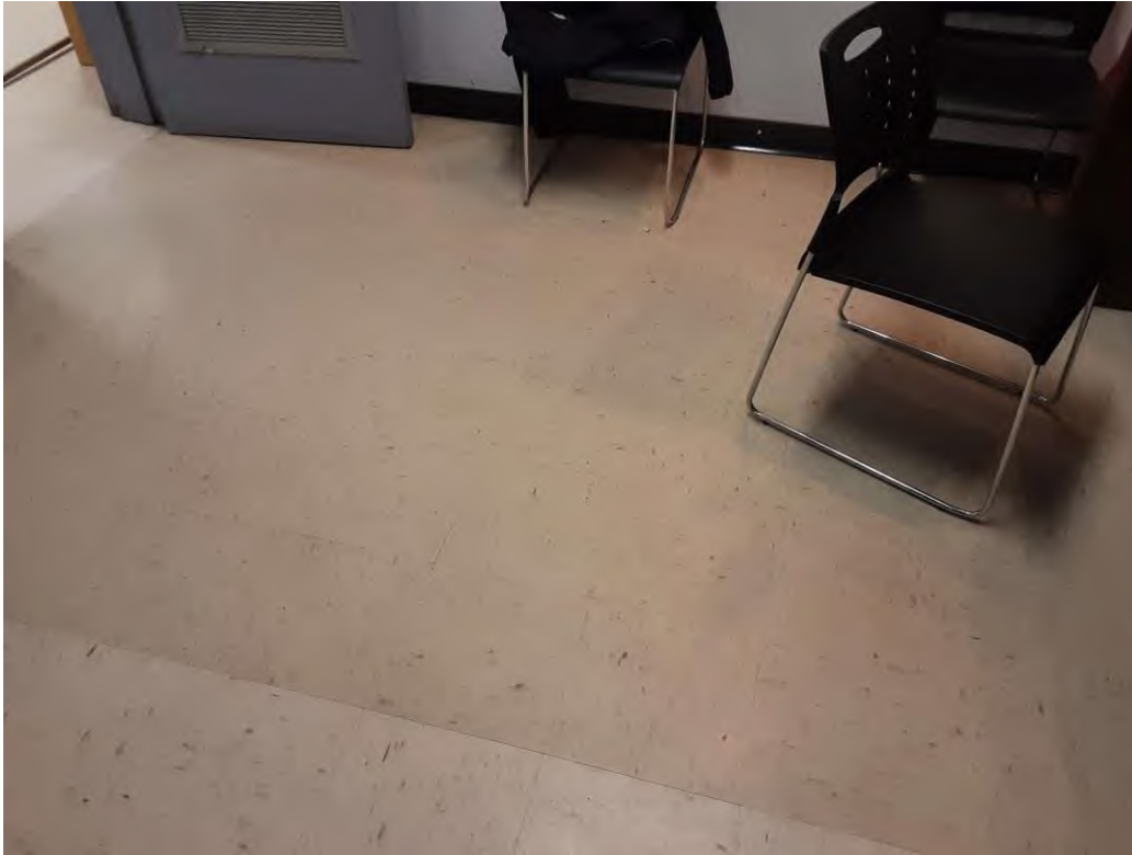
S0013A (Confirmed Asbestos), 12" beige with brown flecks, Floor, All, Vinyl Floor Tile and Mastic, Administration Office (Location #: 7)
