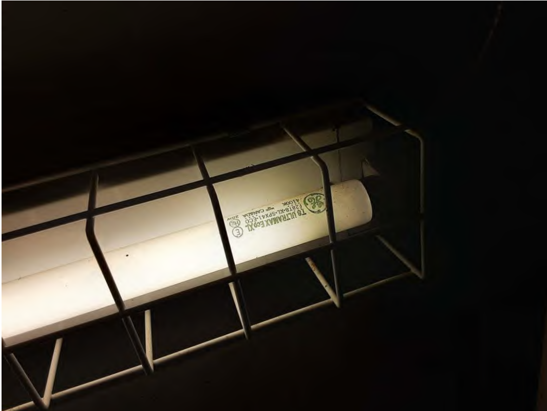
Mercury, V9000(Yes), LIGHT FIXTURE, Boiler Room Storage (Location #: 2)
