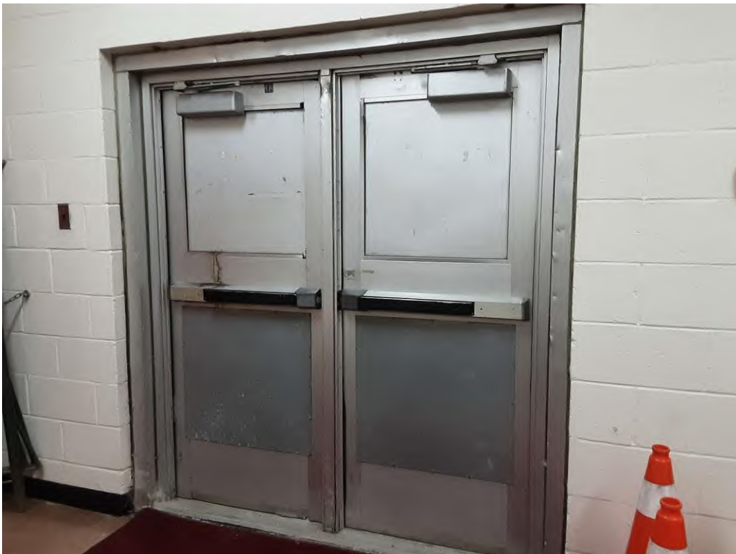
S0021A (Confirmed Asbestos), Grey, Other, Door, Caulking, Gym Vestibule (Location #: 30)
