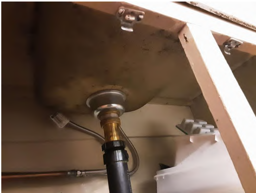
S0018 (Confirmed Asbestos), Other, Sink, Mastic, Gold, Classroom (Location #: 24)
