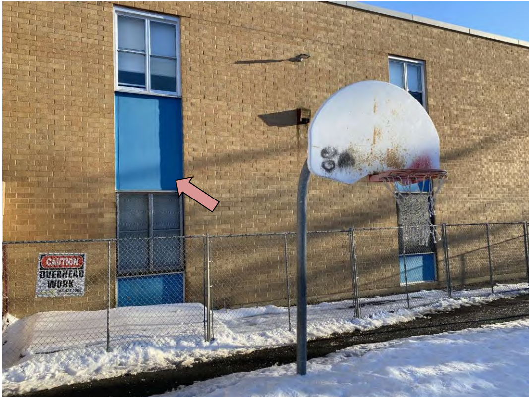
S0031A (Confirmed Asbestos), Transite, Wall, Exterior, Cement Product, Exterior (Location #: 76) Panels around windows painted red and blue. Sampled from previously damaged area
