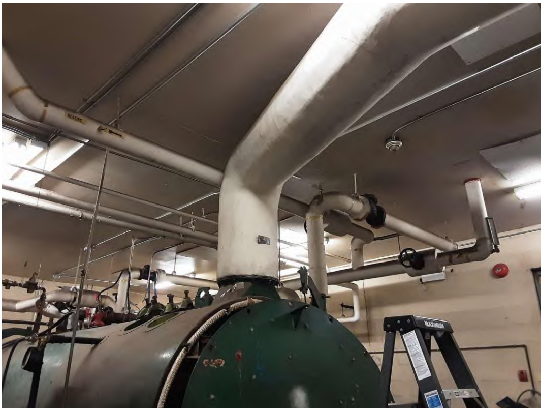
S0003A (Confirmed Asbestos), Duct, Boiler, Parging Cement, Boiler Room (Location #: 1)
