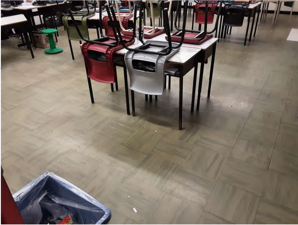
S0025A (Confirmed Asbestos), 12" green with light green streaks, Floor, All, Vinyl Floor Tile and Mastic, Classroom (Location #: 52)
