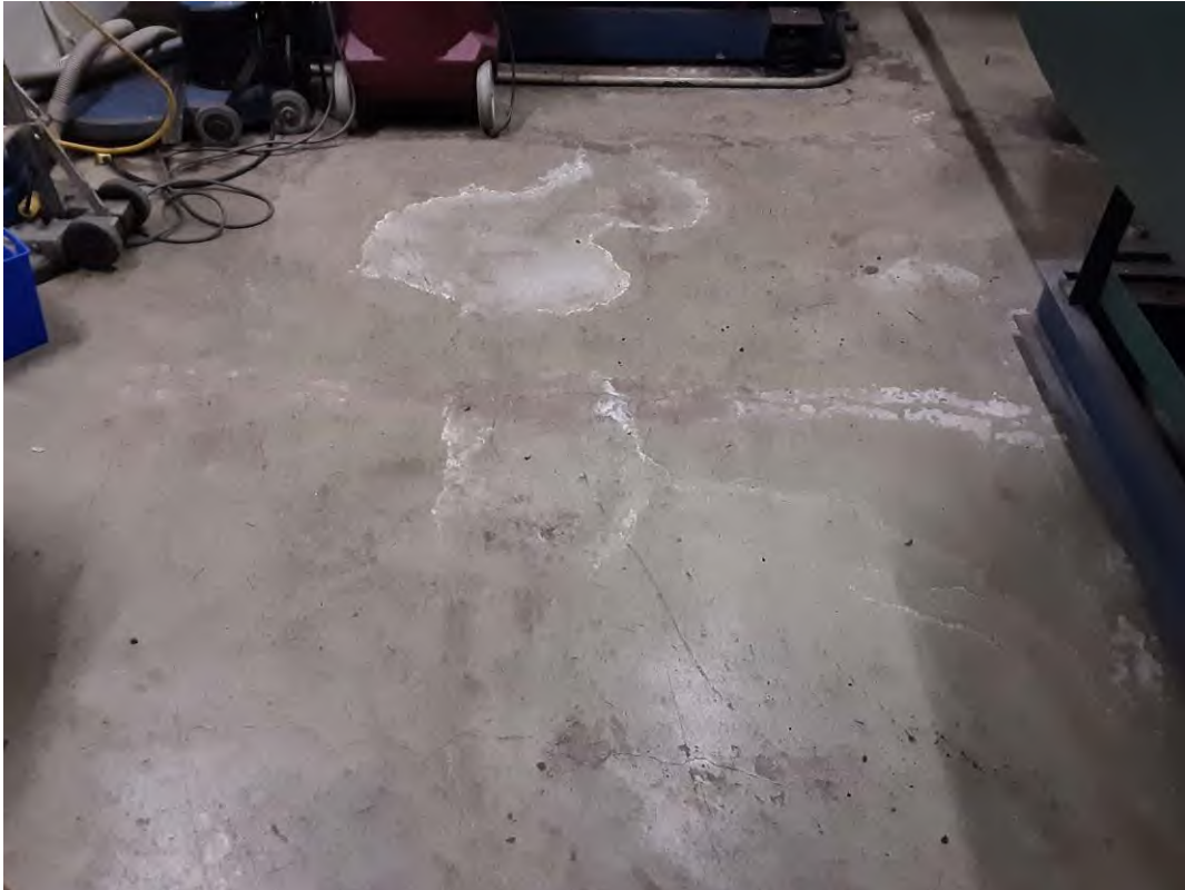
L0008(Lead, High), Green, Floor, Mechanical Room (Location #: 64)
