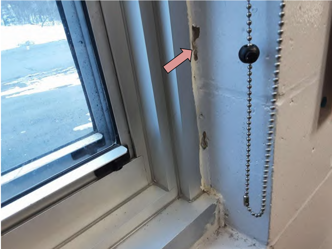
S0010A (Confirmed Asbestos), Grey, Other, Window, Caulking, Principal Office (Location #: 4)
