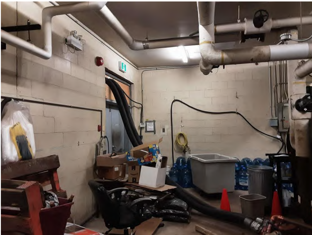
L0001(Lead, High), White, Wall, Boiler Room (Location #: 1)
