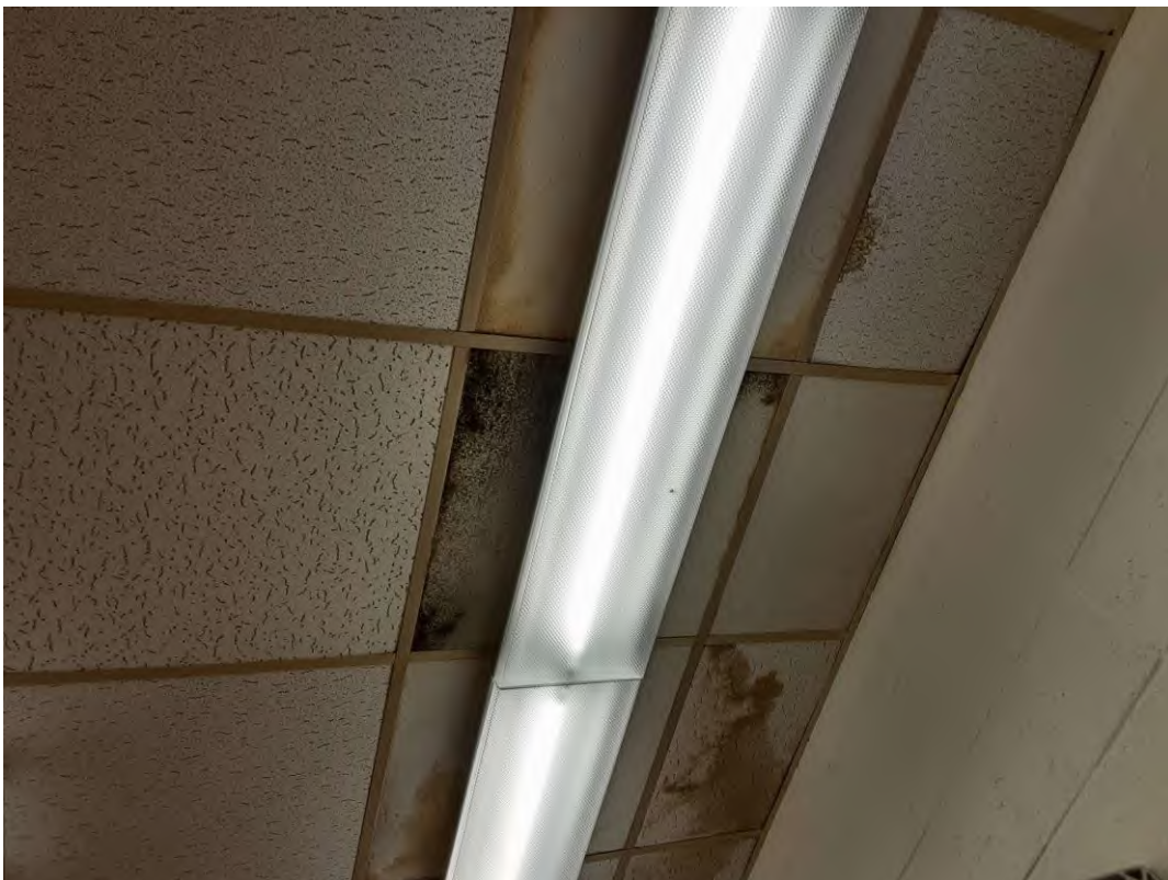
Mould, (Yes), Ceiling, Ceiling Tiles (lay-in), Classroom (Location #: 57) Visible mould growth
