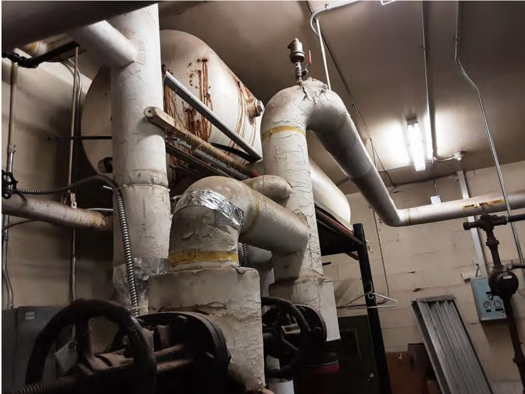
S0001A (Confirmed Asbestos), Piping, Heating Water Supply, Parging Cement, Boiler Room (Location #: 1)
