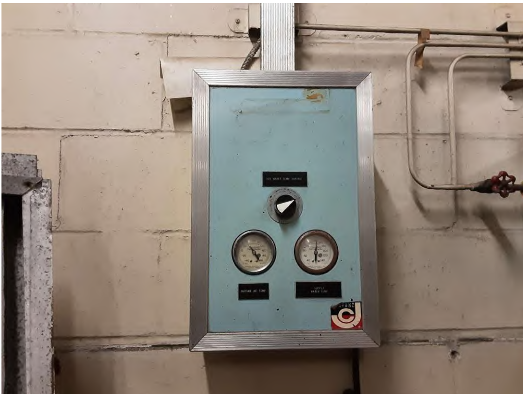
Mercury, V9500(Presumed), BOILER CONTROL, Boiler Room (Location #: 1)
