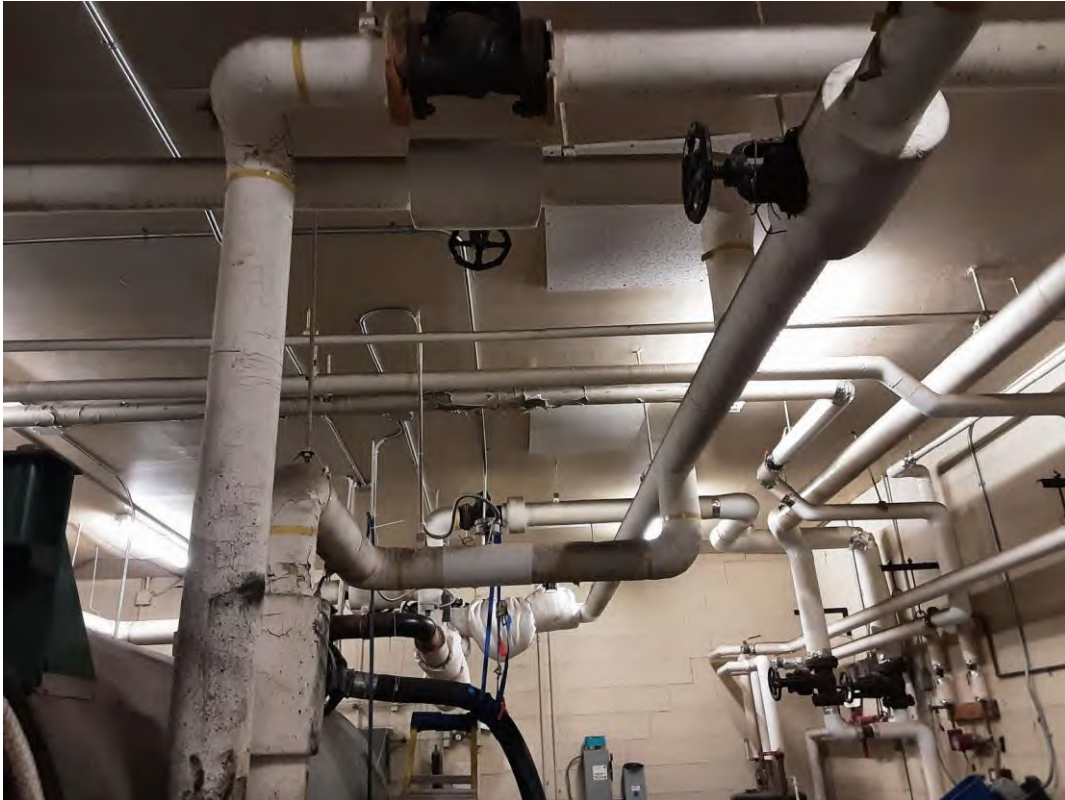
S0004A (Confirmed Asbestos), Piping, Heating Water Return, Parging Cement, Boiler Room (Location #: 1)
