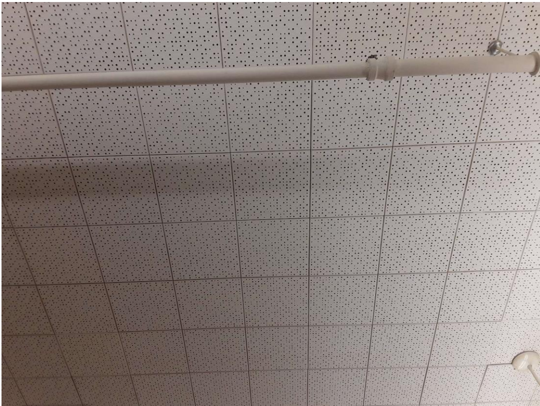
V9500 (Presumed Asbestos), 12"x12", holes, Ceiling, Ceiling tiles (glue-on), Classroom (Location #: 3) Ceiling tiles and mastic are presumed asbestos-containing.
