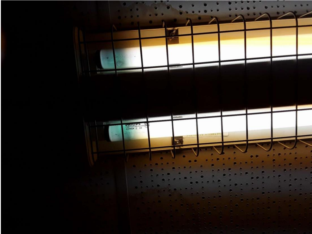
PCB, V9500 (Presumed), LIGHT BALLASTS, Storage (Location #: 16) Ballasts associated with T12 fixtures.
