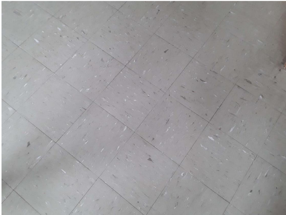
S0021A (Confirmed Asbestos), 9" pale green with white and grey flecks, Floor, Vinyl Floor Tile and Mastic, Gym Office and Storage (Location #: 14)
