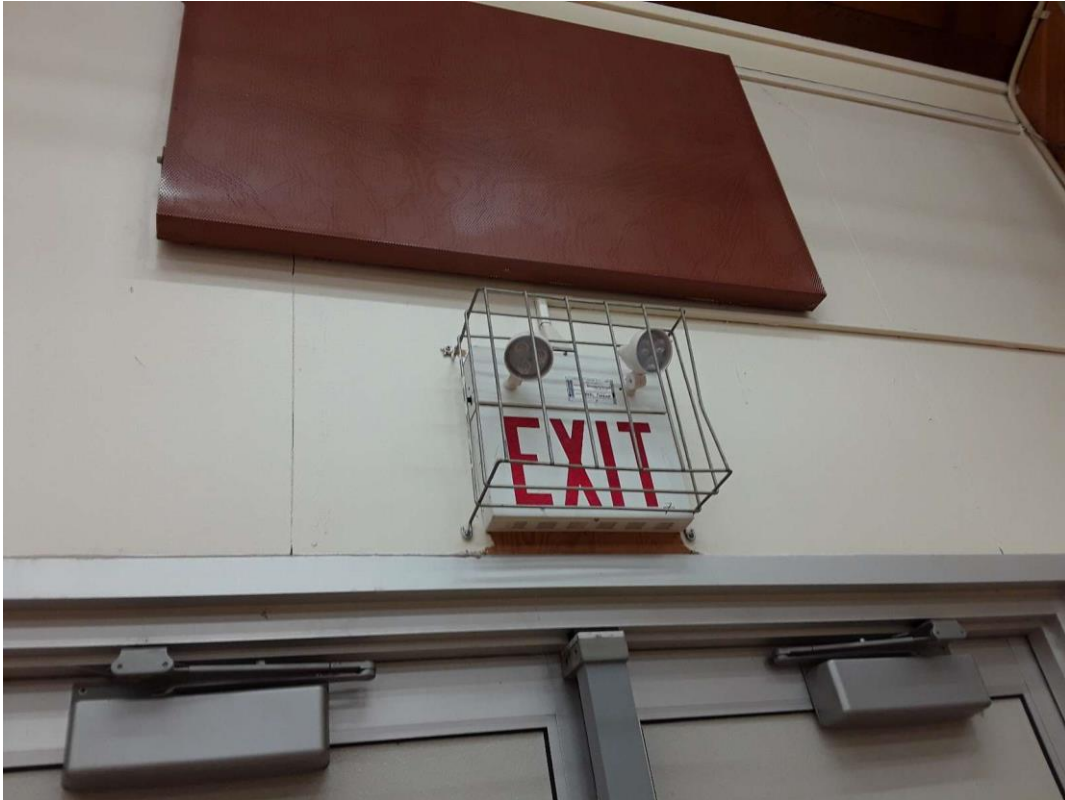
Lead Products, V9500 (Presumed), Batteries in Emer. Lights, Gymnasium (Location #: 13)
