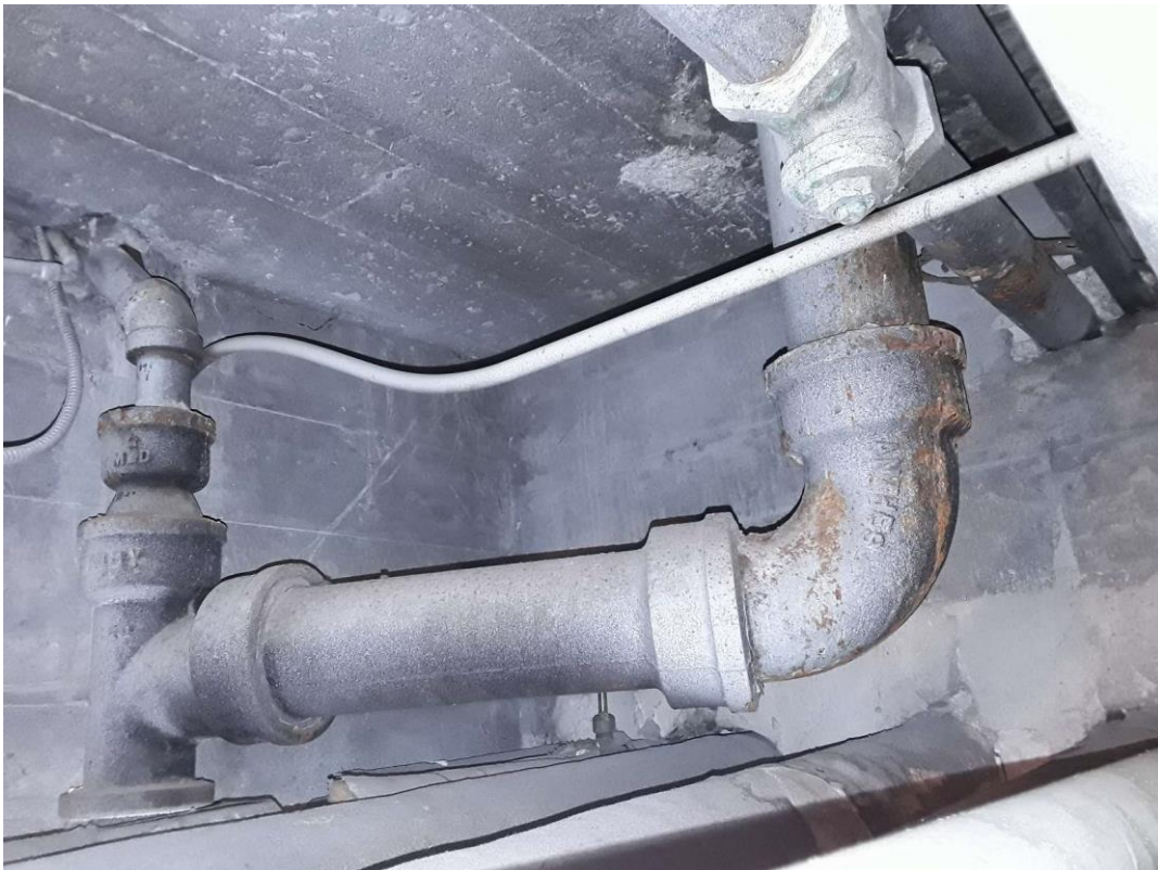
Lead Products, V9000 (Yes), BELL AND SPIGOT FITTINGS, Electrical Room (Location #: 7)
