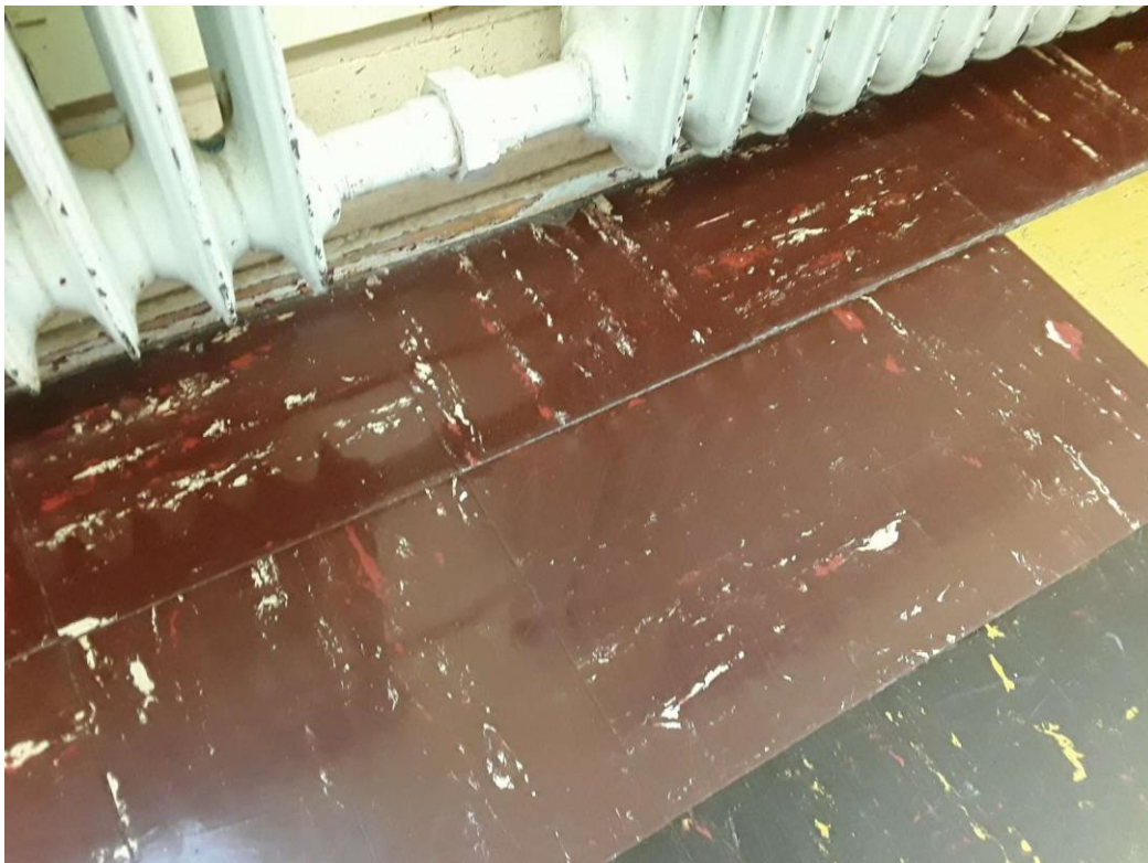
S0038A (Confirmed Asbestos), 9" dark red with white streaks, Floor, Vinyl Floor Tile and Mastic, Classroom (Location #: 33)
