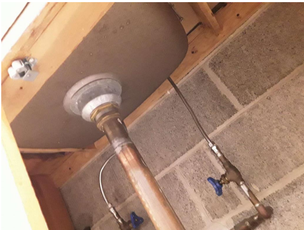
S0011 (Confirmed Asbestos), Other, Sink, Mastic, Gold, Staff Room (Location #: 5)
