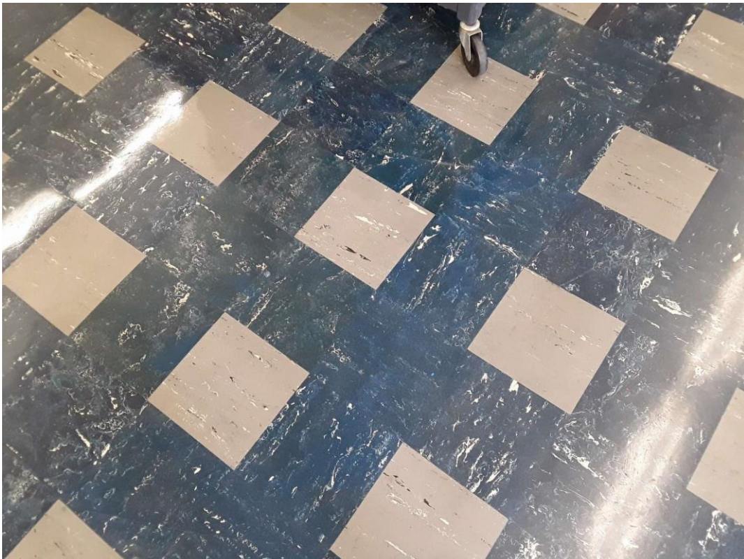
S0034A (Confirmed Asbestos), 9" dark blue and white marble, Floor, Vinyl Floor Tile and Mastic, Classroom (Location #: 32)
