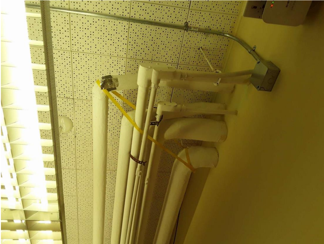
V0004 (Confirmed Asbestos), Piping, Hot Water Heating, Parging Cement, Classroom (Location #: 12)
