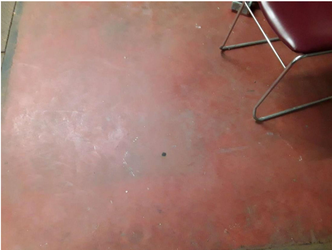
L0001 (Lead, Low), Red, Floor, Boiler Room (Location #: 1)
