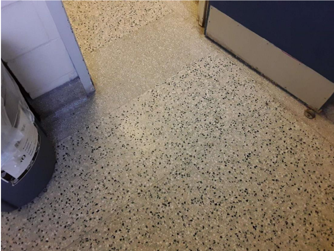
V9500 (Presumed Asbestos), Floor, Terrazzo, Girls Washroom (Location #: 18)
