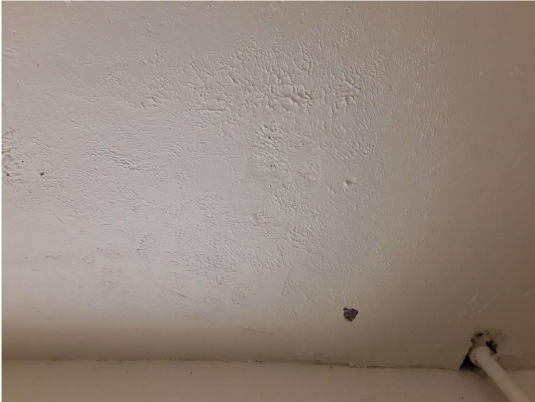
S0016A (Confirmed Asbestos), Ceiling, Plaster, Girls Washroom (Location #: 8)
