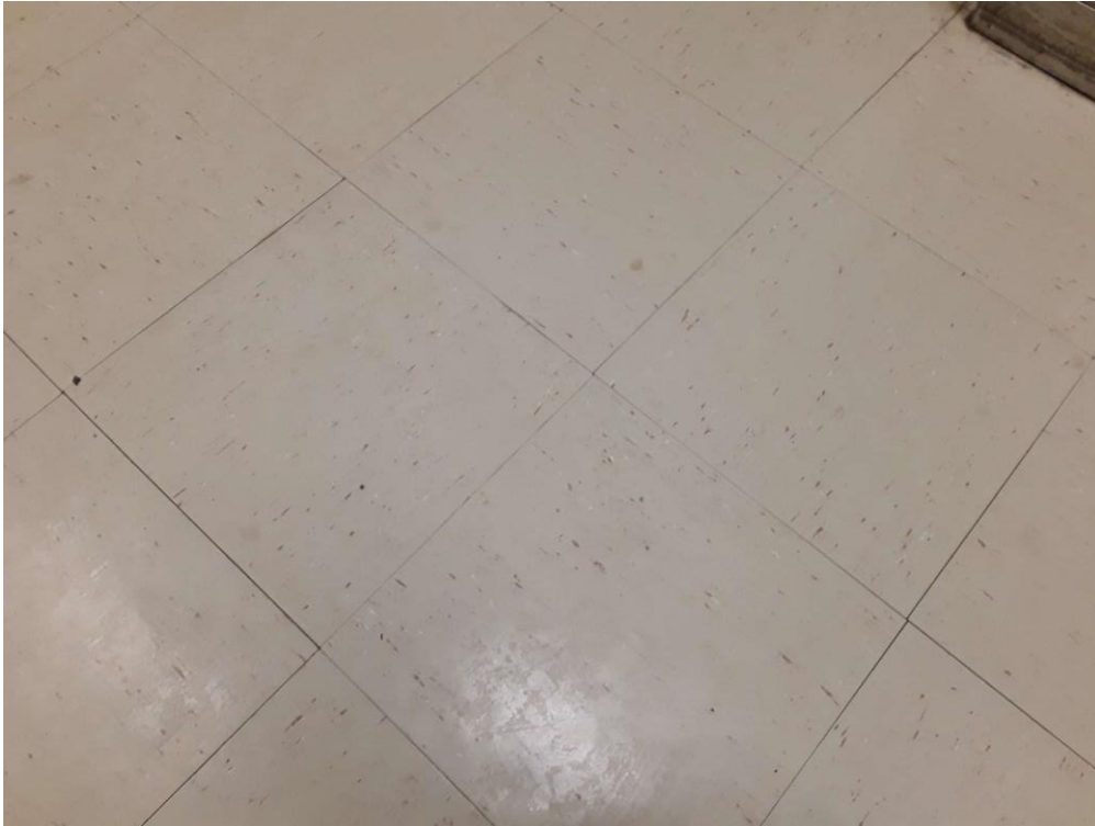
S0013A (Confirmed Asbestos), 12" beige with white and brown flecks, Floor, Vinyl Floor Tile and Mastic, Boys Washroom (Location #: 6)
