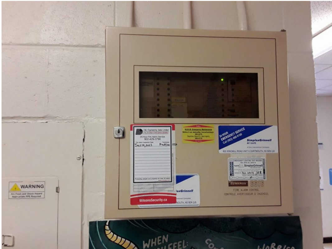
Lead Products, V9500 (Presumed), BATTERIES (OTHER), Hallway and Main Entrance (Location #: 29)
