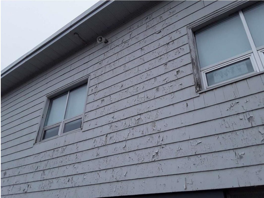
L0008 (Lead, High), White, Wall, Exterior (Location #: 46)
