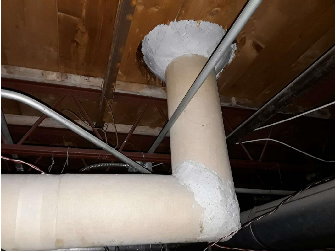
S0033A (Confirmed Asbestos), Piping, Roof Hopper (Drain), Parging Cement, Hallway and Main Entrance (Location #: 29)
