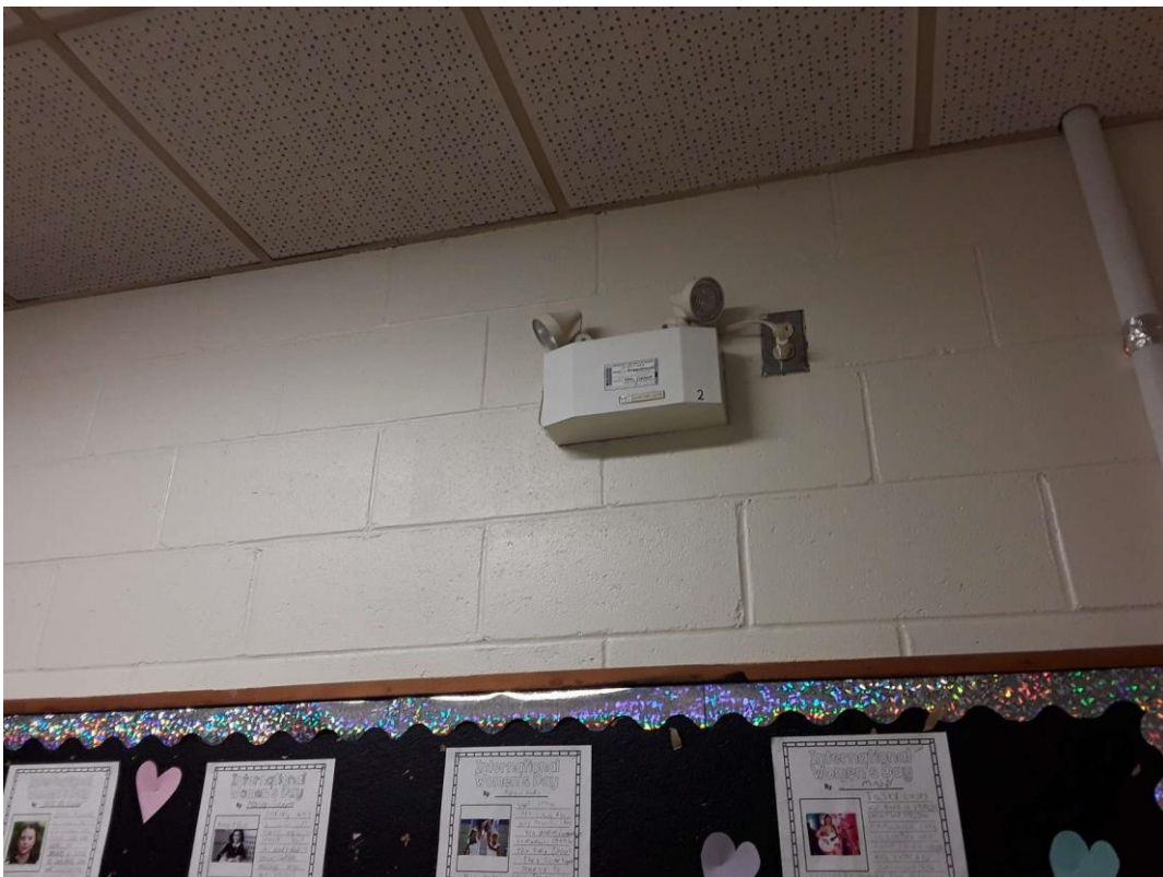
Lead Products, V9500 (Presumed), BATTERIES IN EMER. LIGHTS, Hallway and Main Entrance (Location #: 29)
