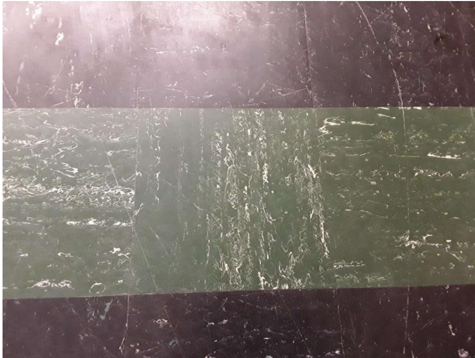
S0043A (Confirmed Asbestos), 9" dark green with white streaks, Floor, Vinyl Floor Tile and Mastic, Classroom (Location #: 40)
