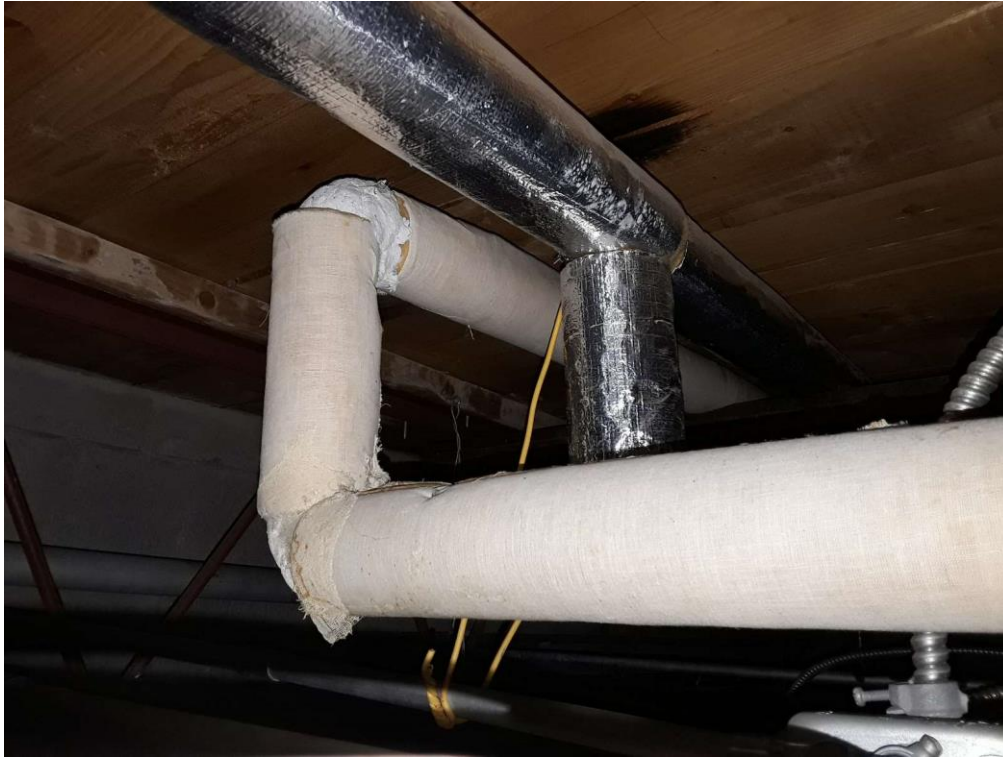
S0023A (Confirmed Asbestos), Piping, Domestic Water (Hot and Cold), Parging Cement, Storage (Location #: 16)
