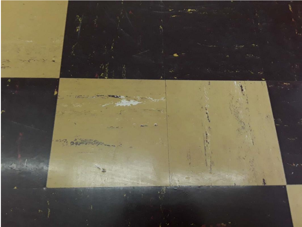
S0037A (Confirmed Asbestos), 9" mustard with white and dark purple streaks, Floor, Vinyl Floor Tile and Mastic, Classroom (Location #: 33)
