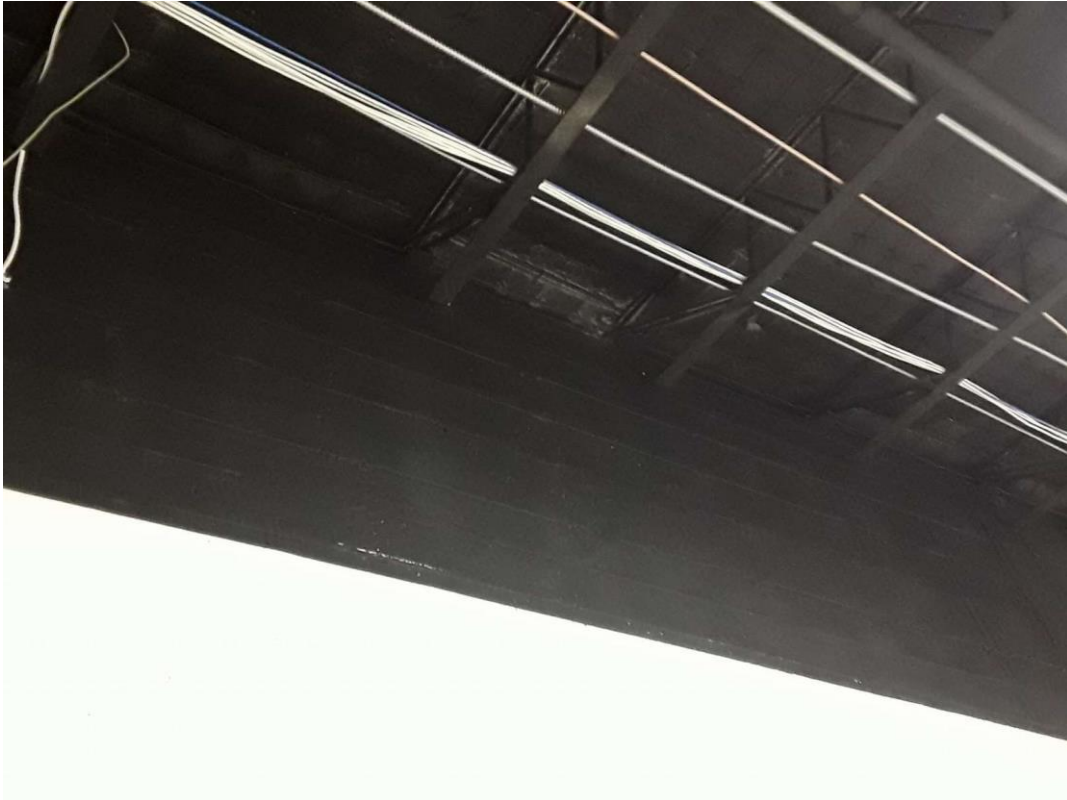
L0012 (Lead, Low), Black, Wall, Hallway (Location #: 31)
