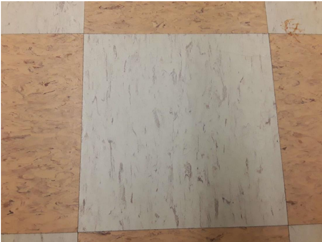
S0018A and S0019A (Confirmed Asbestos), 9" cream with brown streaks and 9" orange with brown streaks, Floor, Vinyl Floor Tile and Mastic, Classroom (Location #: 11)
