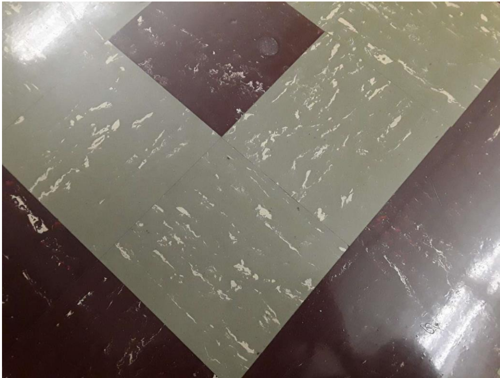
S0041A (Confirmed Asbestos), 9" pale green with white streaks, Floor, Vinyl Floor Tile and Mastic, Classroom (Location #: 38)
