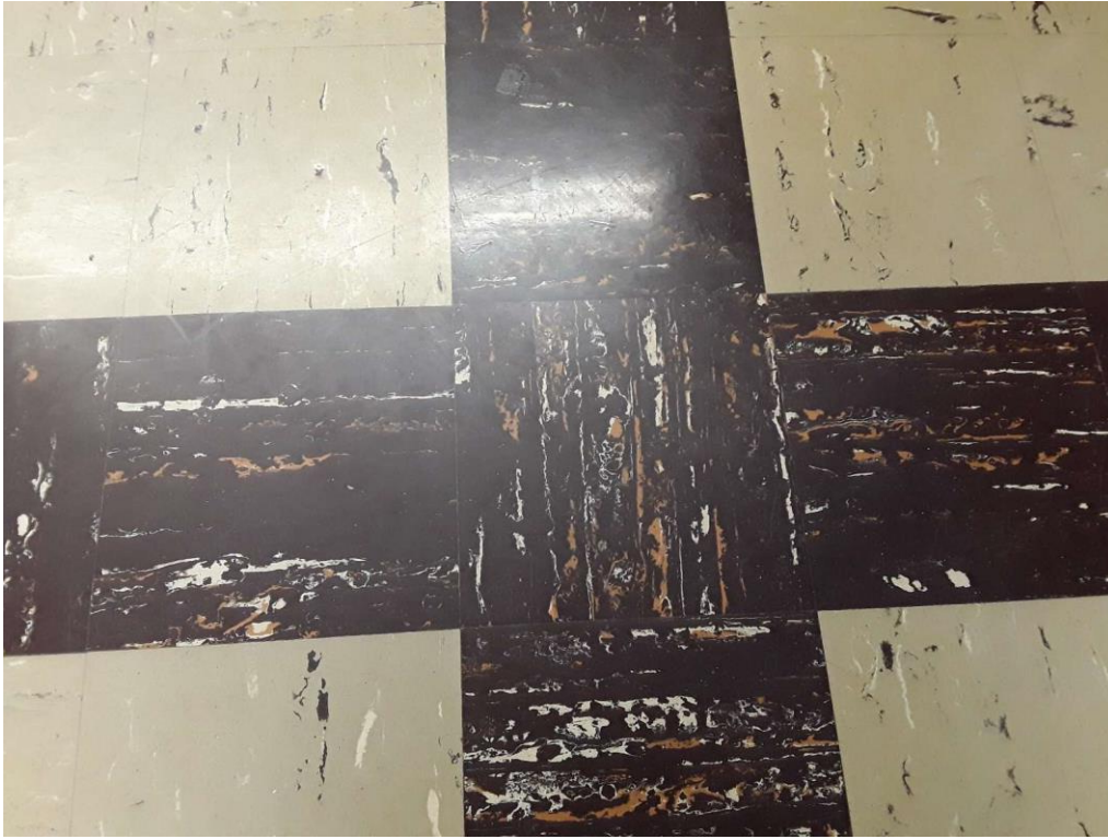
S0039A (Confirmed Asbestos), 9" dark brown with white and orange streaks, Floor, Vinyl Floor Tile and Mastic, Library (Location #: 35)
