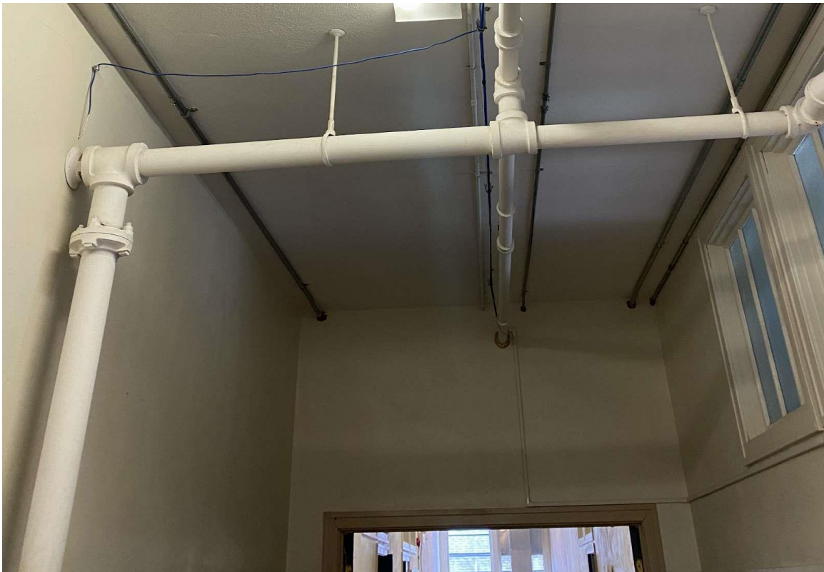
S0016G (Confirmed Asbestos), Wall, Interior, Plaster, Hallway (Location #: 42)
