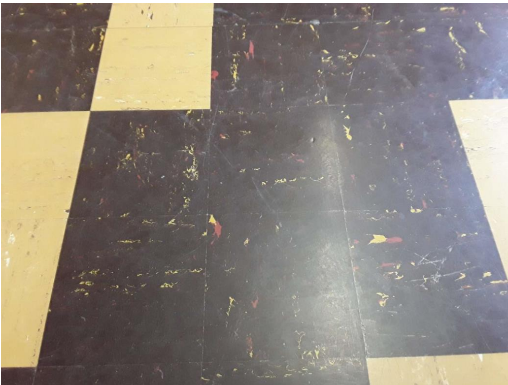
S0036A (Confirmed Asbestos), 9" dark purple with red and yellow streaks, Floor, Vinyl Floor Tile and Mastic, Classroom (Location #: 33)
