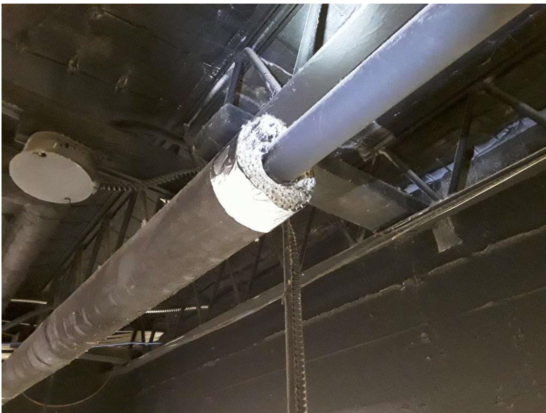
S0003B (Confirmed Asbestos), Piping, Hot Water Heating, Aircell, Hallway (Location #: 31) Canvas painted black
