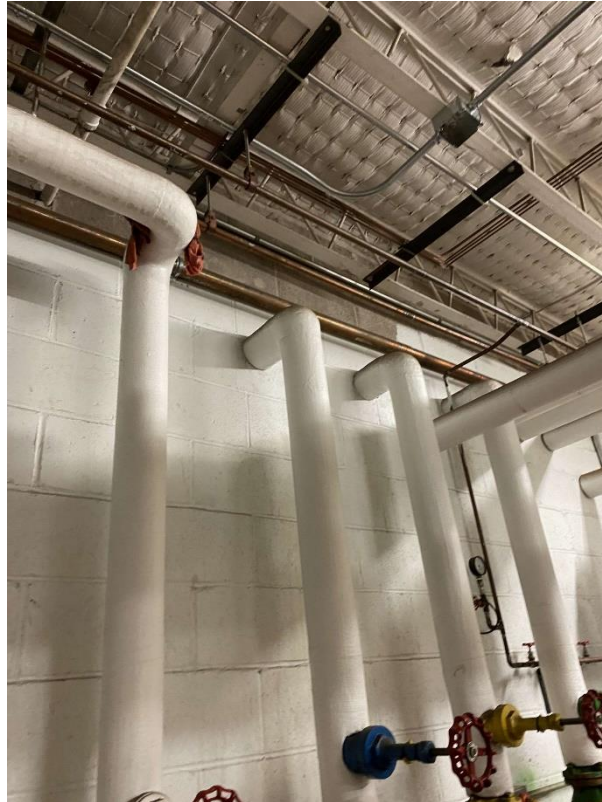
S0002B (Considered Asbestos), Piping, Hot Water Heating, Parging Cement, Boiler Room (Location #: 1) Considered asbestos-containing unless additional sampling completed.
