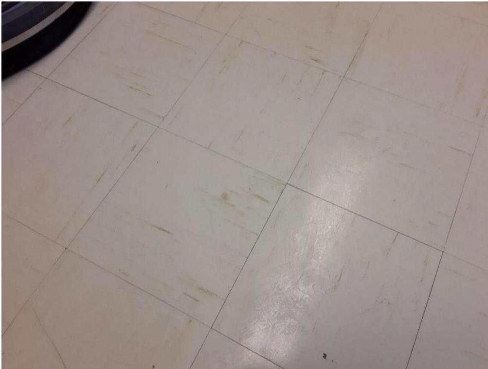
S0024A (Confirmed Asbestos), 9" off-white with green streaks, Floor, Vinyl Floor Tile and Mastic, Caretaker Office (Location #: 17)
