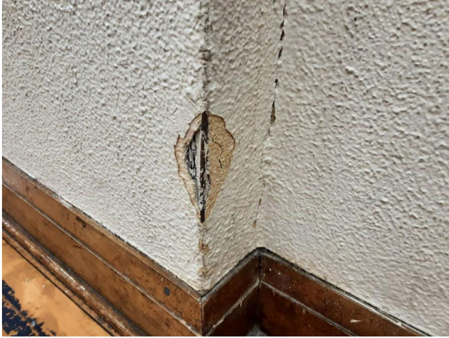
Confirmed Asbestos, S0001A-G, Wall, Plaster, Gym (Location #: 7)
