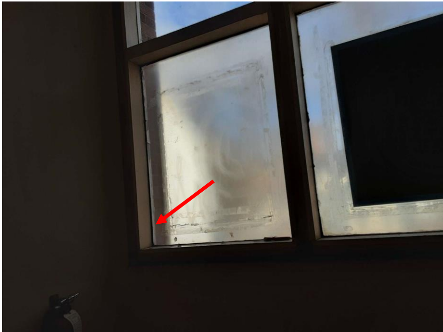
Confirmed Asbestos, S0007A-C (Confirmed Asbestos), Window, Black Butyl Tape, Vestibule 1 (Location #: 5)
