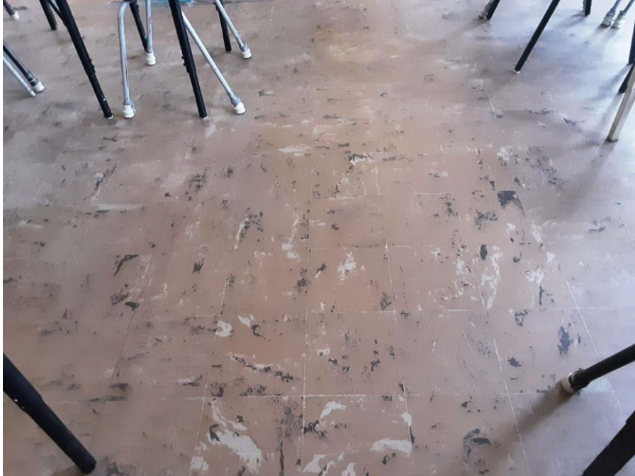
Confirmed Asbestos, S0011A-C, Floor, Vinyl Floor Tile and Mastic, Classroom 2 (Location #: 16) 9" Brown Marble Pattern
