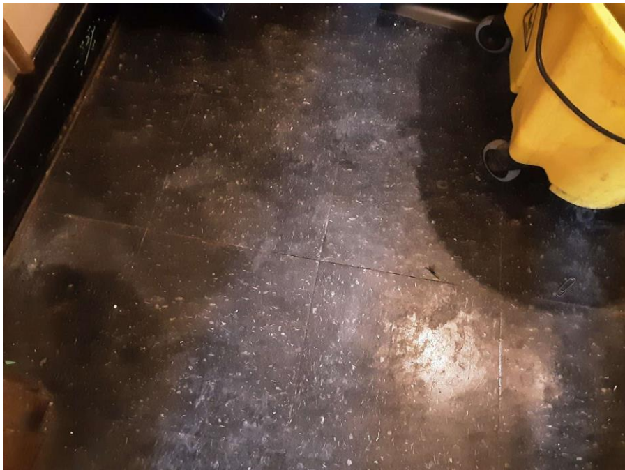
Confirmed Asbestos, S0010A-C, Floor, Vinyl Floor Tile and Mastic, Maintenance Room (Location #: 14) 12" Black
