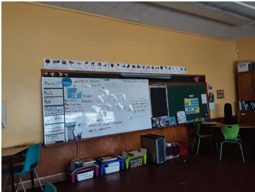
L0004(Lead (High)), Plaster, Yellow, Classroom 1 (Location #: 15)
