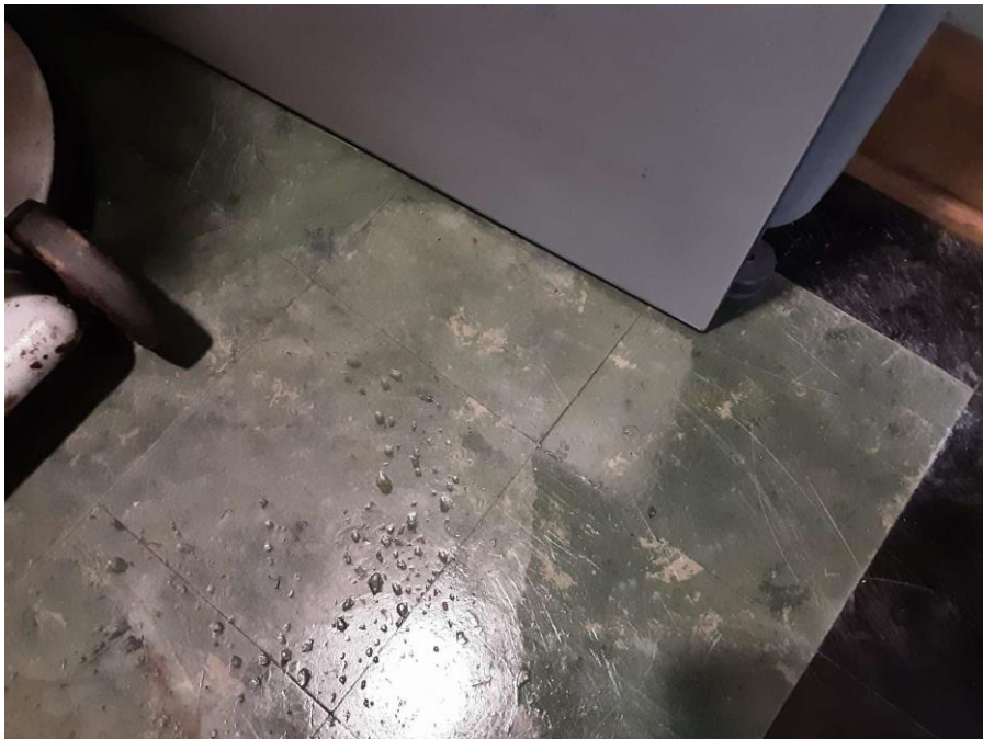
Confirmed Asbestos, S0012A-C, Floor, Vinyl Floor Tile and Mastic, Storage Closet 2 (Location #: 17) 9" Green
