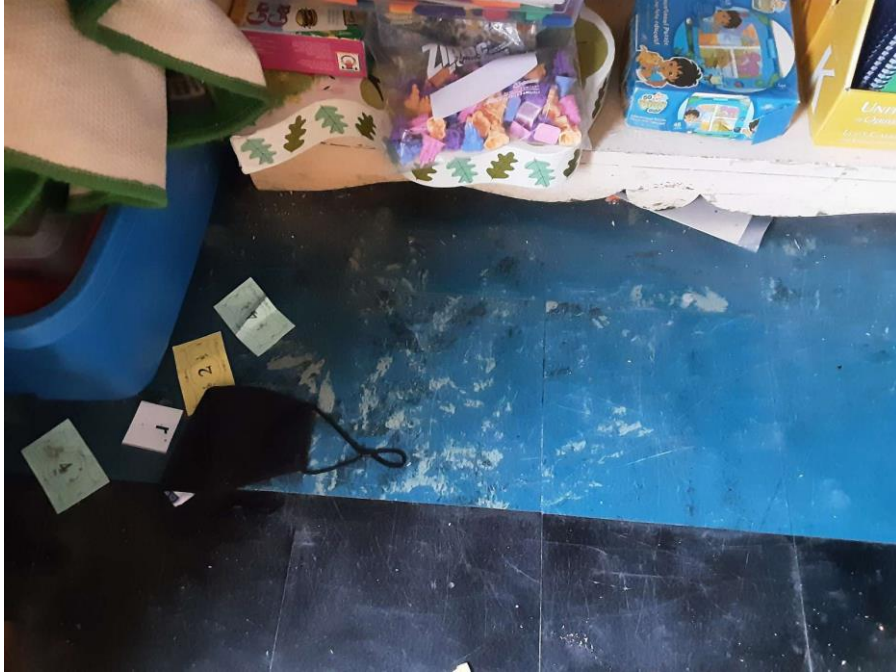
Confirmed Asbestos, S0019A-C, Floor, Vinyl Floor Tile and Mastic, Classroom 5 Closet (Location #: 29) 9" Teal Marble Pattern
