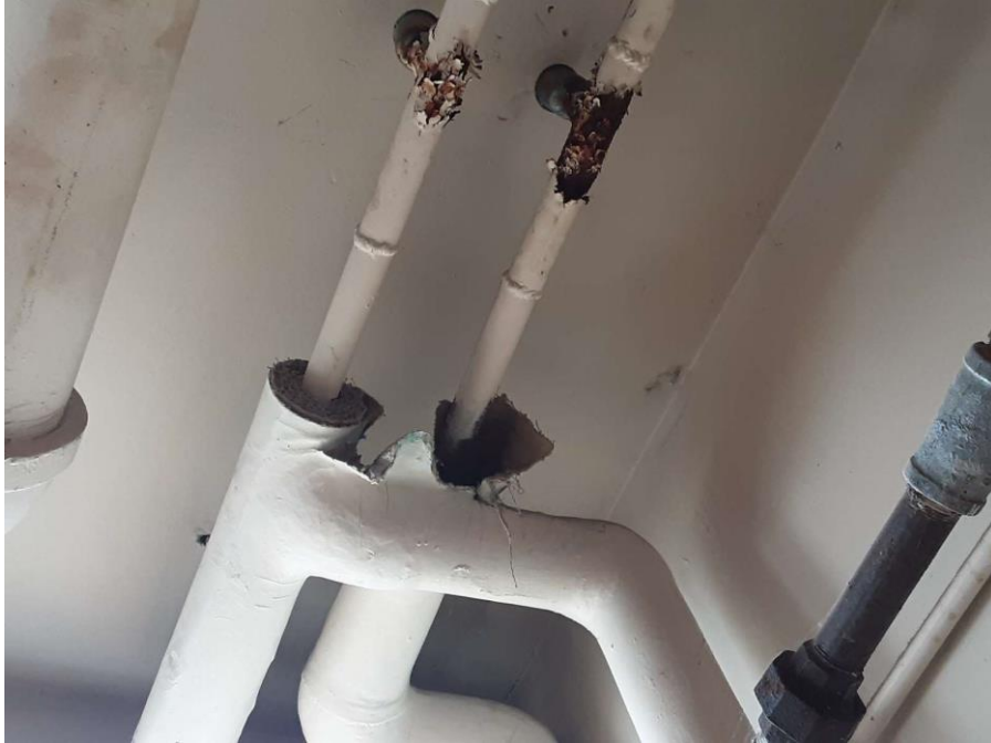
Confirmed Asbestos, S0006A-C, Piping, Heating Water Supply, Aircell, Sprinkler Room (Location #: 3)
