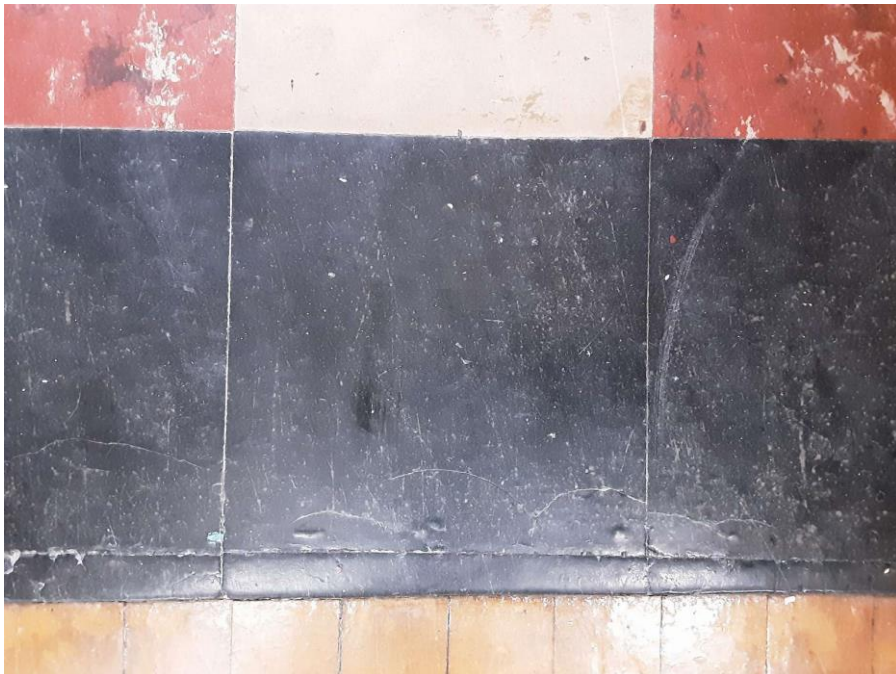
Confirmed Asbestos, S0005A-C, Floor, Vinyl Floor Tile and Mastic, Sprinkler Room (Location #: 3) 9" Black
