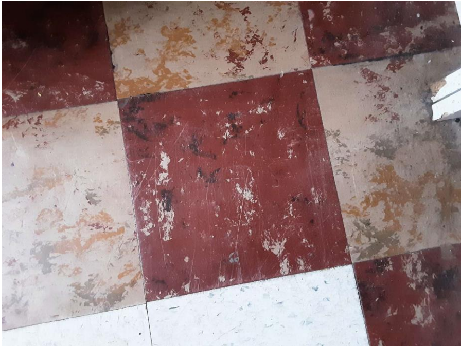
Confirmed Asbestos, S0003A-C, Floor, Vinyl Floor Tile and Mastic, Sprinkler Room (Location #: 3) 9" Red Marble Pattern
