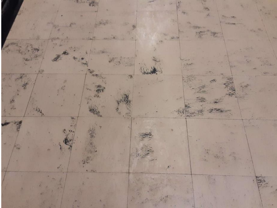
Confirmed Asbestos, S0009A-C, Floor, Vinyl Floor Tile and Mastic, Hallway Ground Floor (Location #: 8) 9" Tan and Black
