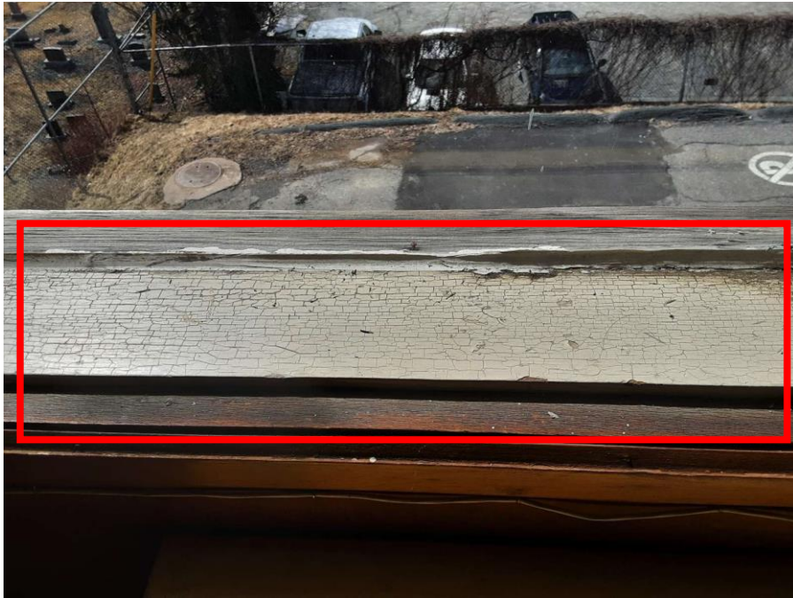
L0005(Lead (High)), Wood, Light yellow, Classroom 3 (Location #: 21)
