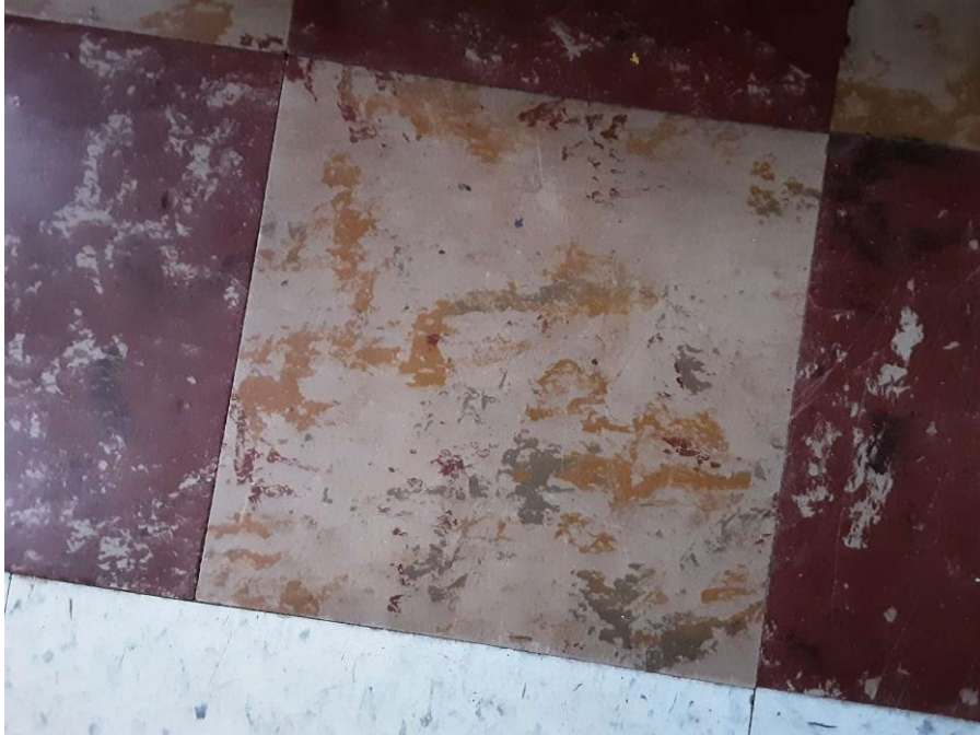
Confirmed Asbestos, S0004A-C, Floor, Vinyl Floor Tile and Mastic, Sprinkler Room (Location #: 3) 9" Beige Marble Pattern
