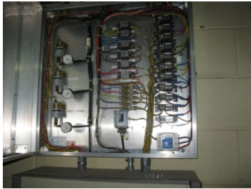
4.7.4 | Control panel in boiler room
