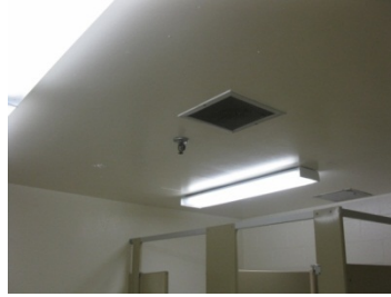
4.6.20 | Washroom exhaust grille
