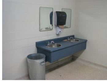
2.5.2 | Upgraded sinks in Female W/C
