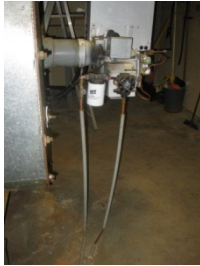
4.4.7 | Oil lines across floor to burner
