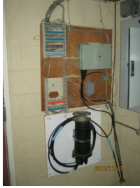
3.5.1 | Communications service entrance
