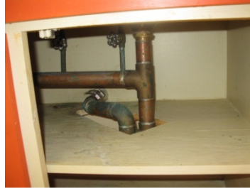
4.3.14 | Kitchen sink with copper drain
