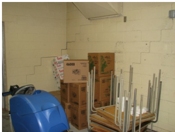
1.2.4 | Cracked concrete block at Level 1 – SW corner
