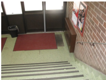
4.5.4 | Entrance Cabinet Heater
