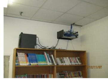
3.5.3 | Network switch in Library
