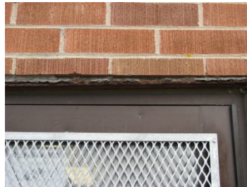
1.4.2 | Deteriorating Steel lintel at West exit doors
