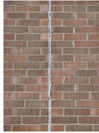
1.2.2 | Failed brick expansion joint
