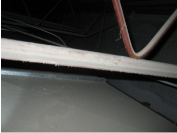
4.6.7 | Dust in Return air plenum
