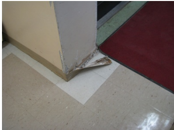
2.3.1 | damage to drywall partition at elevator alcove
