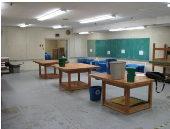
2.1.7 | Painted concrete floor requiring painting
