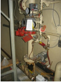
4.8.1 | Sprinkler alarm valve in boiler room
