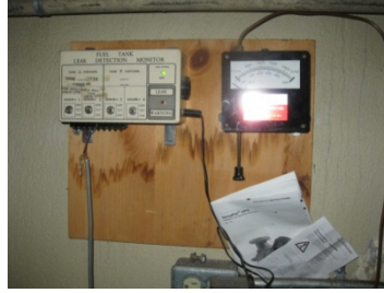
4.4.5 | Oil Tank monitor and gauge
