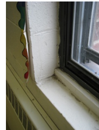
1.3.3 | Evidence of water leakage at classroom windows
