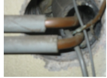
4.4.6 | Oil lines from underground oil tank
