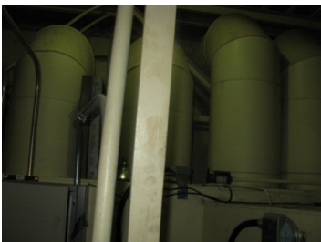
4.6.16 | AH-3 supply ducts
