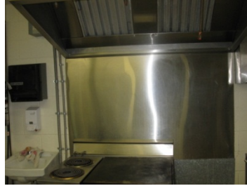
4.6.23 | Current exhaust hood
