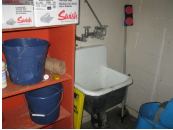
4.3.13 | Service Sink with no vacuum breaker
