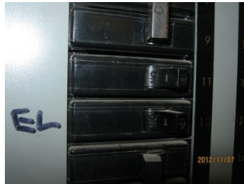
3.1.8 | Panel 'P4' (Emergency Light Battery Breaker)
