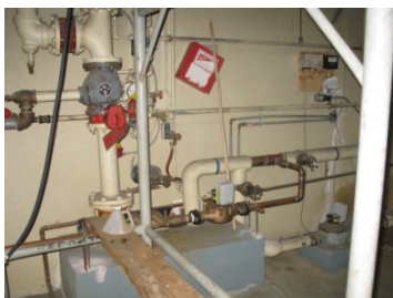
4.1.1 | Sprinkler Domestic Water Entrance
