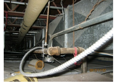
3.1.12 | Wiring installed in Ceiling Space
