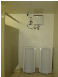
4.3.4 | Flush tank Urinals with occupancy sensor
