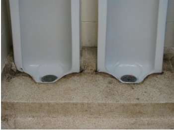
2.1.4 | Terrazzo floor very dirty around urinals
