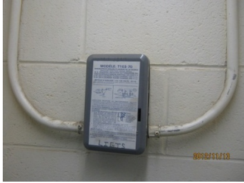
3.2.10 | Exterior lighting time clock
