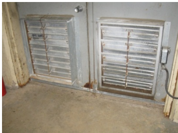
4.6.25 | Boiler room combustion air
