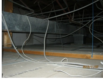
3.1.11 | Wiring Installed in Ceiling Space
