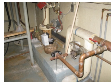
4.1.3 | Sprinkler Domestic Water Entrance
