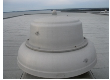
4.6.21 | Typical roof mounted exhaust fan
