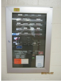
3.4.1 | Custom 6500 Fire Alarm panel
