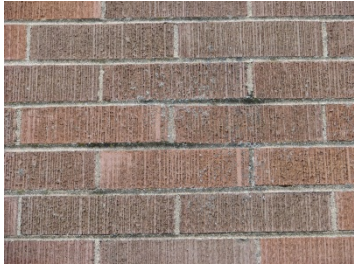
1.2.1 | Deteriorating mortar joints on the south façade
