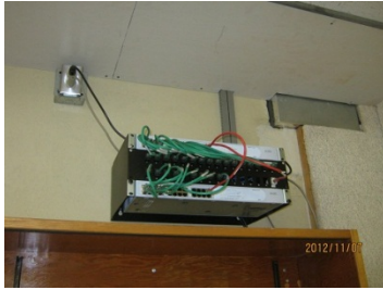
3.5.4 | Network switch in Computer Room
