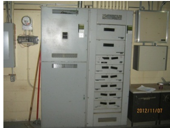
3.1.2 | Main Service Entrance Switchboard
