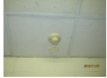
3.4.3 | Fire Alarm smoke detector
