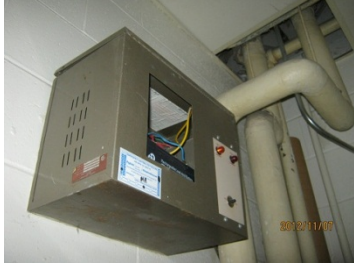
3.3.4 | Remote emergency battery unit
