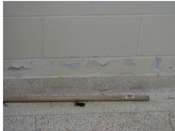
2.3.2 | Peeling paint on concrete block in Change Room 236
