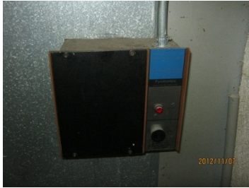
3.4.4 | Fire Alarm duct mounted smoke detector
