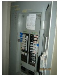
3.1.5 | Panel 'D' (Missing Panel Directory)
