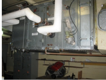
4.6.8 | AH-2 in boiler room
