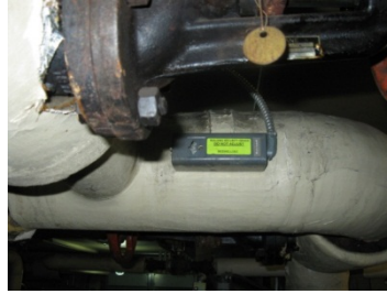
4.7.2 | Control panel in boiler room
