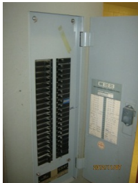
3.1.7 | Panel 'P1' (No Spare Breakers)
