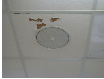
2.2.5 | Damaged 24"x24" ceiling tiles
