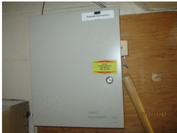
3.8.1 | Security System Panel
