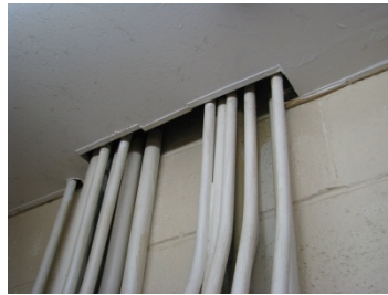
2.2.8 | Penetration through fire rated ceiling
