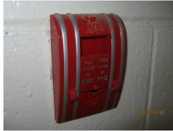
3.4.5 | Pull station missing glass rod
