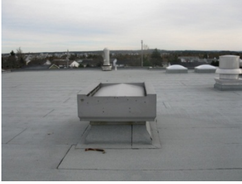
4.6.4 | Relief hood on roof
