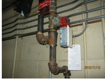
4.8.2 | Elevator Supervised valve in boiler room
