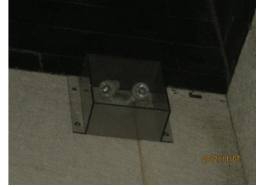
3.3.3 | Gymnasium emergency light
