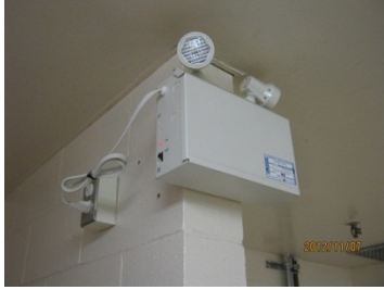
3.3.1 | Typical emergency lighting unit
