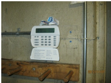
3.8.4 | Keypad in Boiler Room
