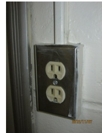
3.1.9 | Surface Raceway and Receptacle
