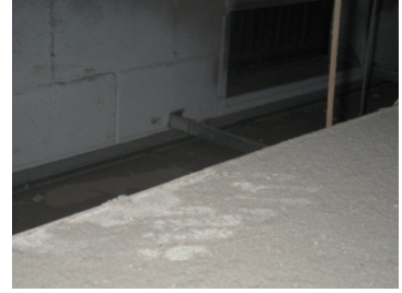
4.6.6 | Return air grille open to the R/A plenum
