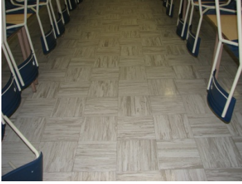
2.1.1 | Original VAT in Cafeteria
