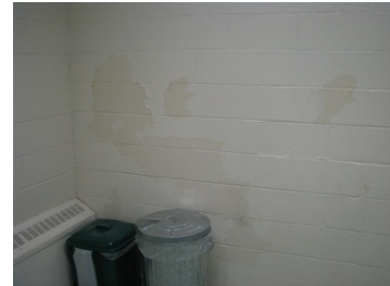
2.3.3 | Peeling paint on concrete block in Stair 306
