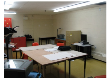
2.2.3 | 2'x4' fissure acoustic tile
