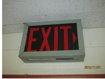
3.3.5 | Typical exit sign
