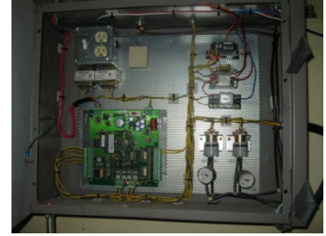
4.7.3 | BAS Control Panel
