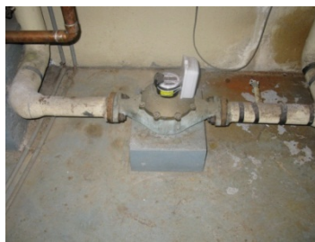
4.1.2 | Domestic Water Entrance
