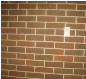
4.7.7 | Aspirating Thermostat for Vestibule
