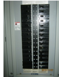
3.1.3 | Panel 'NE' (Added for Elevator Equipment)
