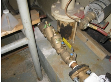
4.1.4 | Backflow preventer for exterior connection for outside activities
