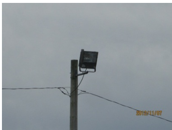
3.2.7 | Exterior pole mounted HID light fixture
