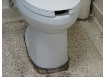
2.1.5 | Terrazzo very dirty around toilets
