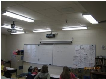
3.2.1 | Typical Classroom lighting
