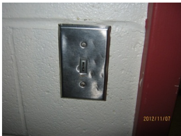
3.2.4 | Washroom key switch
