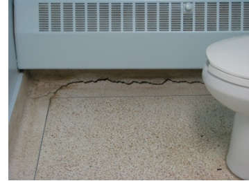
2.1.6 | Significant crack in Admin W/C terrazzo flooring.
