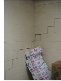
1.2.3 | Cracked concrete block at Level 1 – SW corner
