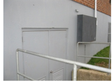
4.6.9 | AH-2 Intake hood
