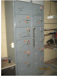
3.1.13 | Motor Control Centre in Boiler Rm.
