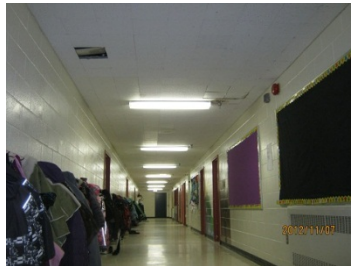
3.2.2 | Typical Corridor lighting
