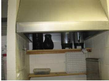
4.6.22 | Original Exhaust hood
