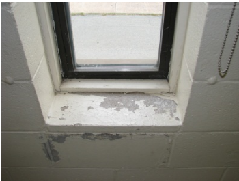
1.3.4 | Evidence of water leakage at cafeteria windows
