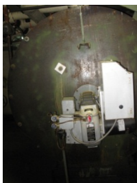
4.4.1 | Oil fired boiler
