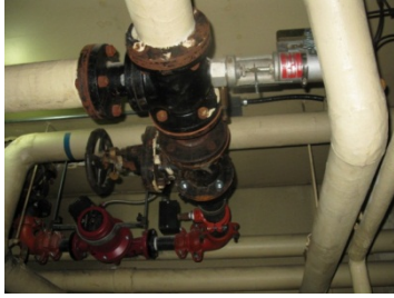
4.4.4 | Circulator and 3 way valve
