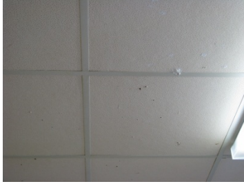
2.2.4 | Marred and, damaged 24"x24" ceiling tiles.
