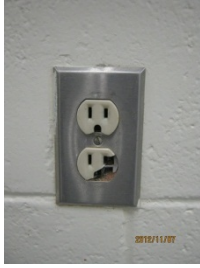
3.1.10 | Receptacle with Damaged Face
