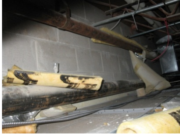
4.5.1 | Heating mains pipe insulation fall off
