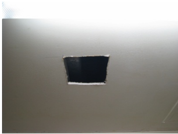
2.2.7 | Hole in GWB ceiling in Female Change Room
