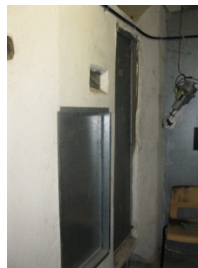
4.6.2 | Built up AH-1 coil and filter sections
