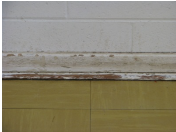
2.3.4 | Wood base in poor condition
