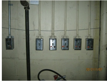
3.1.14 | Manual Motor Starters in Boiler Rm.
