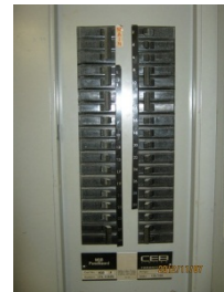
3.1.6 | Panel 'C' (No Spare Breakers)
