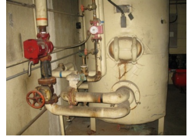
4.1.6 | Domestic Hot water tank with pumps.
