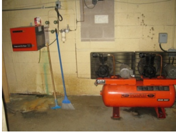
4.7.1 | Control Air Compressor
